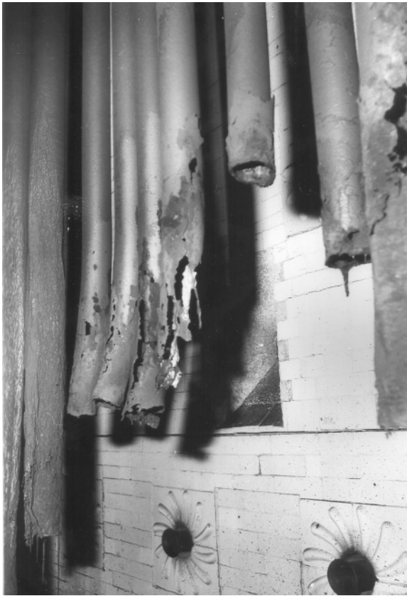
15.3 Overheating failure of radiant tubes.
