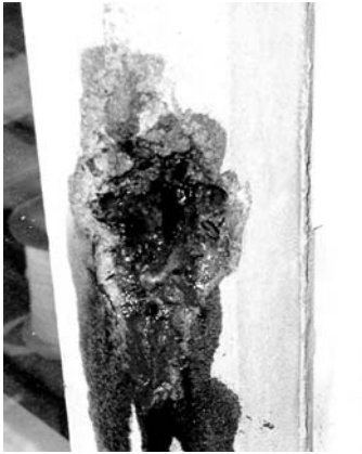
Figure 4.9 Phenolphthalein applied to a concrete window mullion showing approximately 10 mm carbonation depth (clear area at surface) and an uncorroded bar in uncarbonated concrete with a cover depth of approximately 40 mm.
