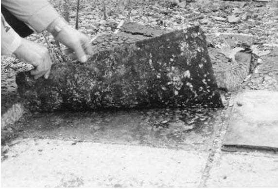
Figure 6.8 Waterproofing membranes can fail to bond, dissolve into the concrete under application of the hot mix wearing course or be punctured by the aggregates. The photograph shows a failed membrane after testing at the UK Transport Research Laboratory.
