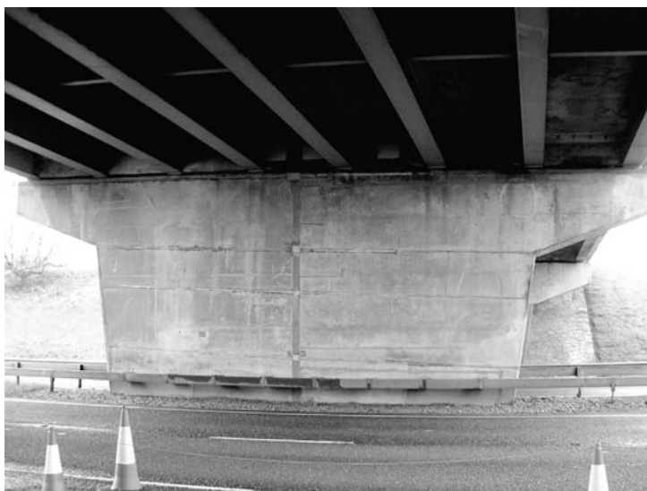
Figure 7.24 A system consisting of wire anodes and cathodes is shown on a bridge in the UK. There are also rod cathodes in the ground drawing water away.
