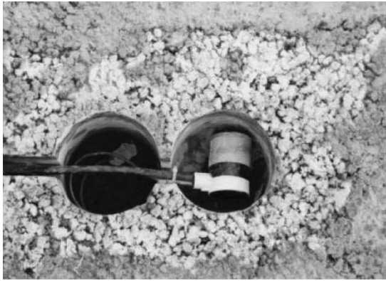
Figure 5.2 A corrosion monitoring probe consisting of a reference electrode and an auxiliary electrode potted up in mortar in the process of installation into a continuously reinforced concrete pavement where corrosion monitoring is required due to the high level of chloride found in the mix water after laying several kilometres of concrete (Broomfield et al. , 2003) photograph. Courtesy BGB Projects Ltd.
