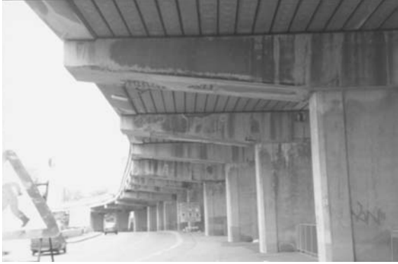
Figure 3.7 The M4 elevated section in West London showing exposed reinforcement due to concrete spalling induced by reinforcement corrosion. Corrosion was caused deicing salt leakage from the deck above.
