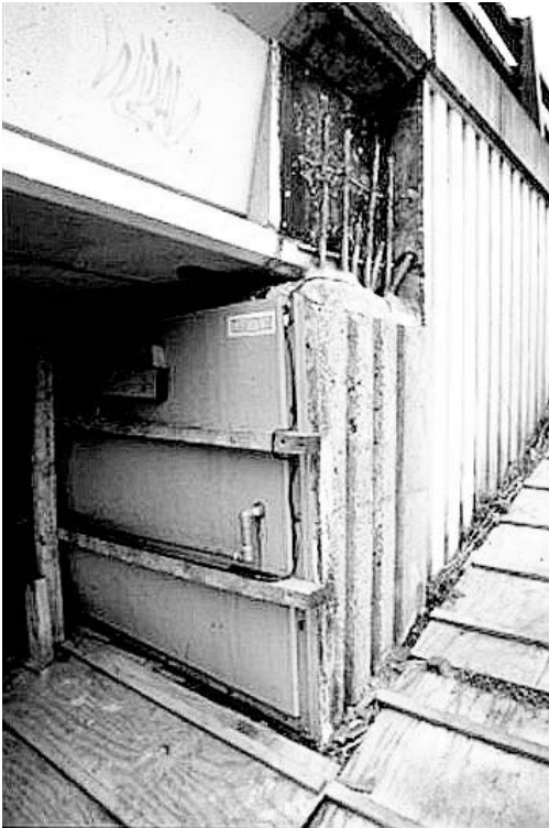
Figure 7.22 Cassette type anode attached to a bridge abutment. Courtesy Makers Ltd.
