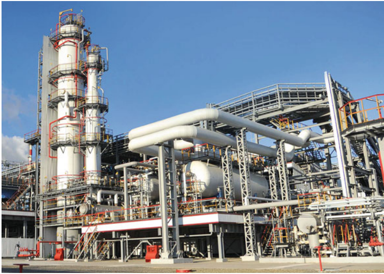
Fig. 1.1 Pipelines—basic component of the oil processing plants CI
