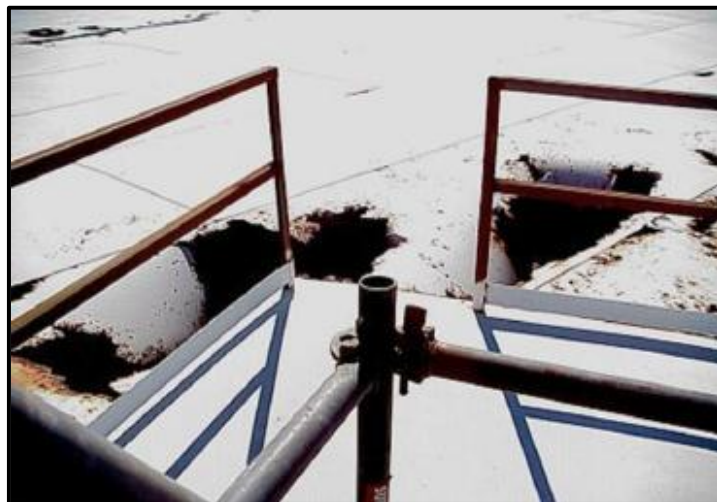
Figure 6 Example of vapour space corrosion
