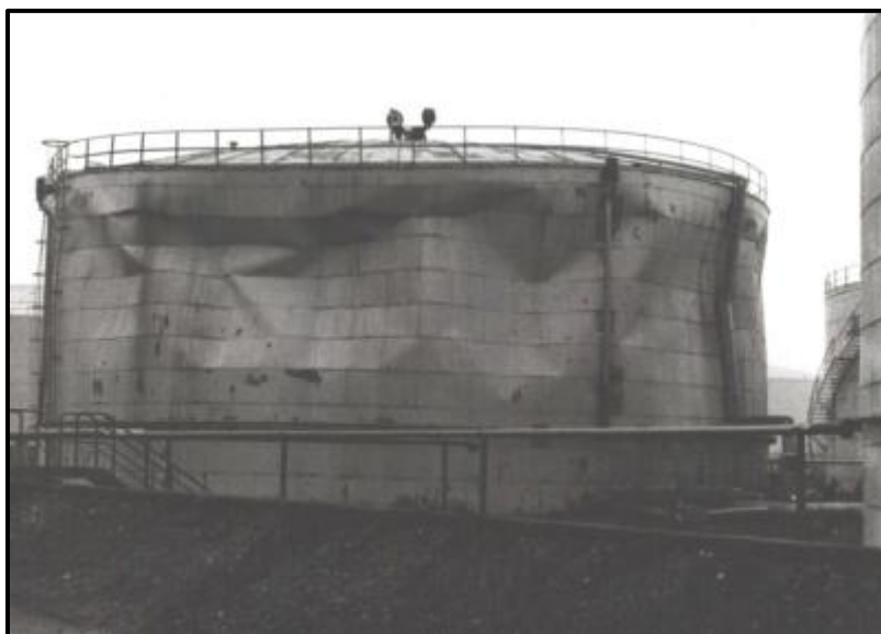
Figure 70 Collapsed fuel tank: vents clogged by frozen rain on the wire mesh
