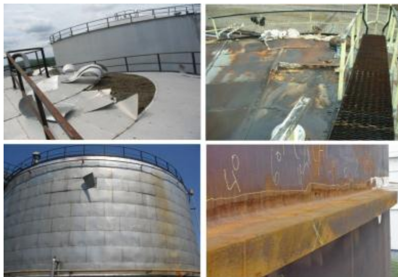
Figure 93 Examples of Corrosion Under Insulation (CUI)
