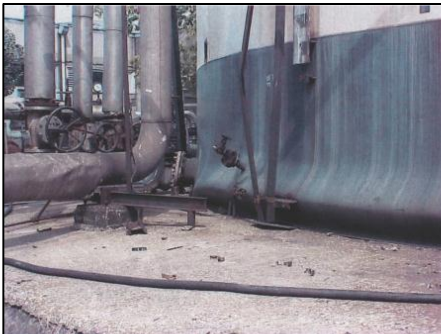
Figure 58 Elephant's foot buckling induced by an earthquake
