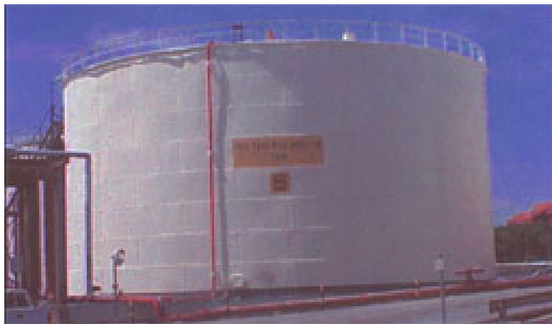
Figure 9 Example of tank built in 1900 and still operational
