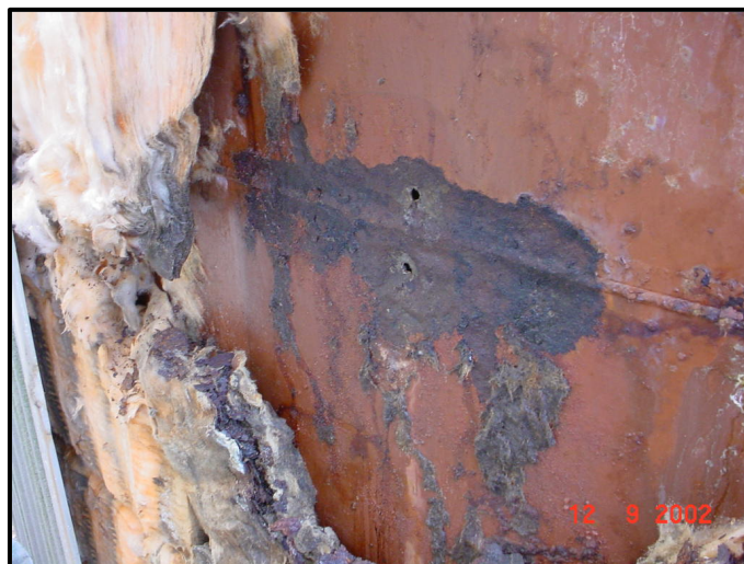
Figure 8 An example of corrosion under insulation
