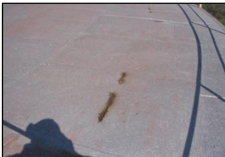
Figure 65 Example of crevice corrosion
