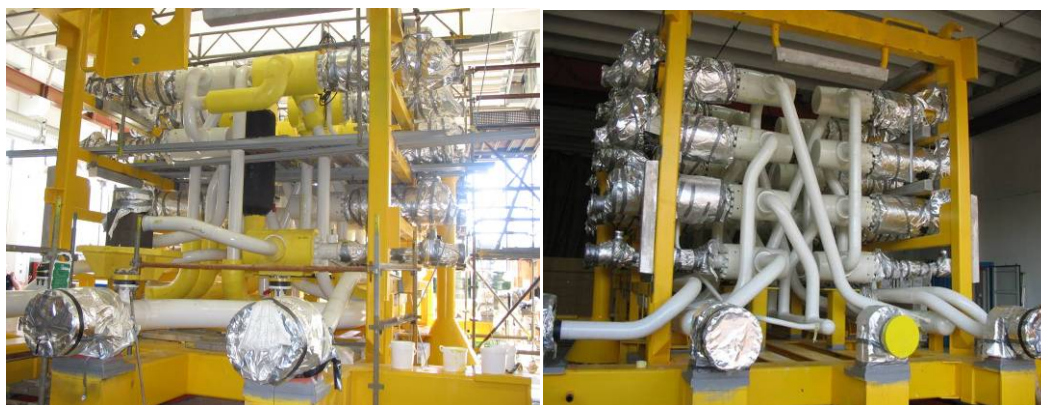
Figure 9 Typical deep water production manifolds during fabrication
