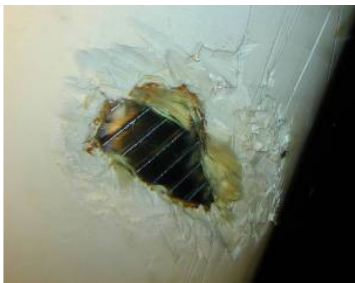
Figure 20 Damaged flexible riser with reinforcing wires exposed
