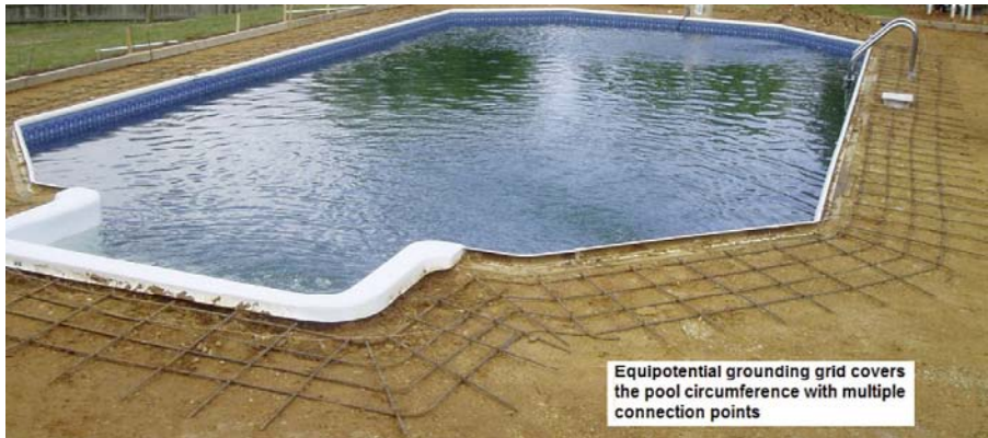
Figure 6.8 An equipotential grounding grid protects anyone getting out of the pool from shock hazards because they would have the same electrical charge as the pad.
