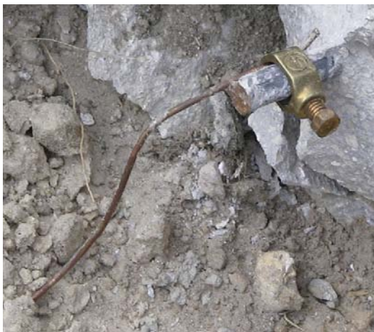
Figure 5.12 A bonding jumper attached to rebar which is encased in concrete.
