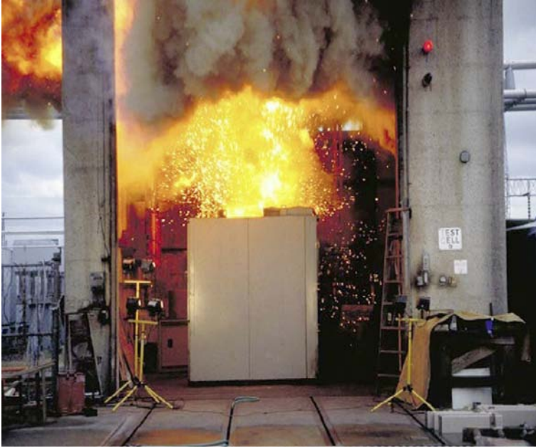
Figure 7.1 An arc blast causes damage from fire, concussion waves, heat, and liquefied metal.
