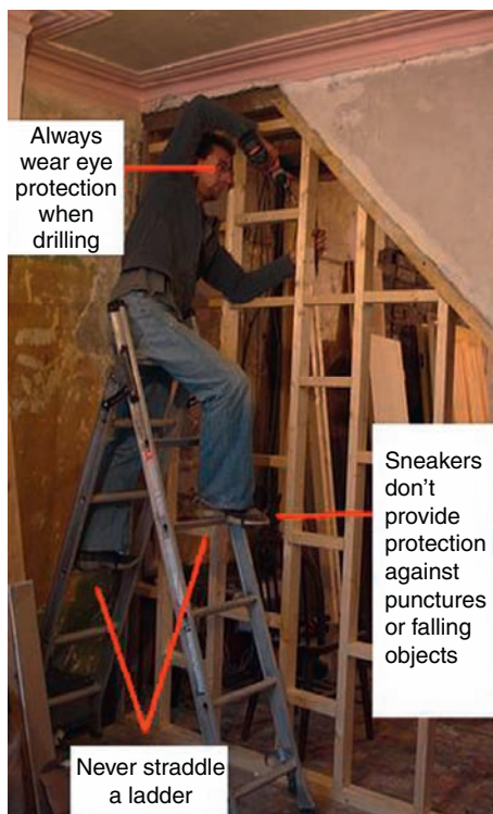
Figure 11.19 Three safety hazards by one worker.
