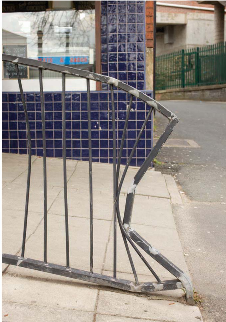
Photo 63 Pedestrian protection railings, showing impact absorbed by vehicle strike, safe plastic deformation of mild steel, even retaining galvanizing corrosion protection, long after damage!
