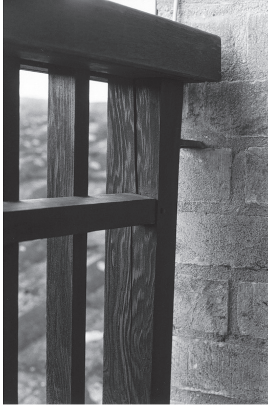
An 18-inch crack in another balustrade.
