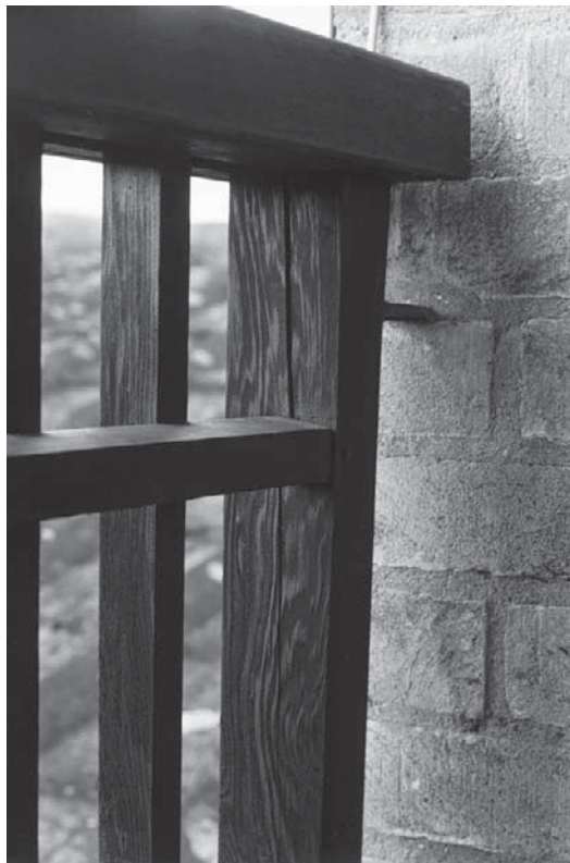
An 18-inch crack in another balustrade.
