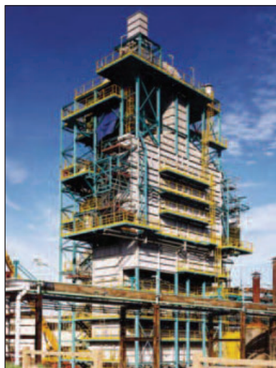
Ethylene Cracker Unit
