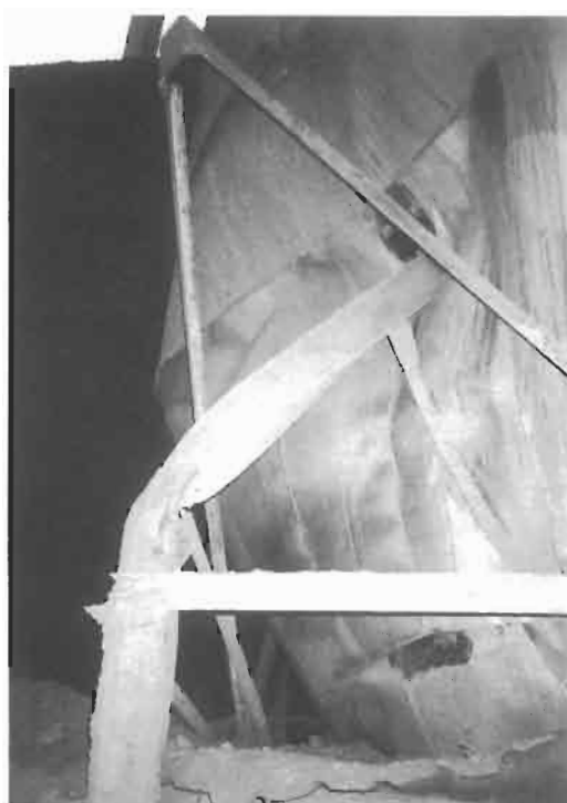
Fig. 3. View of buckled column.
