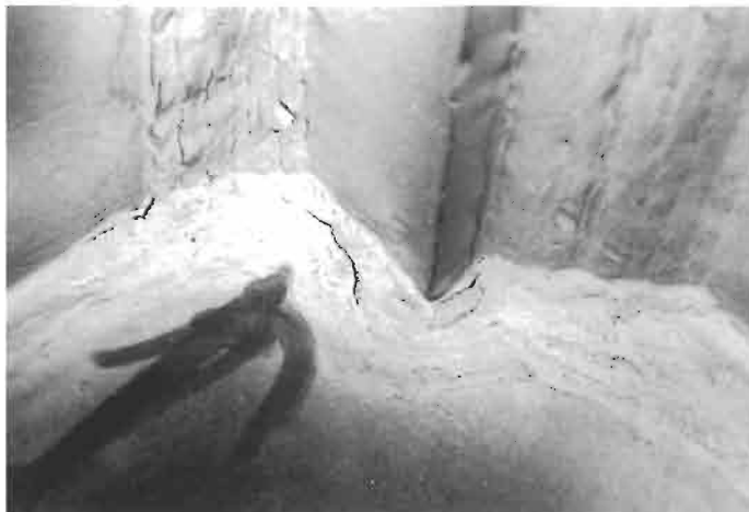
Fig. 4. Typical cracks found at external support welds.
