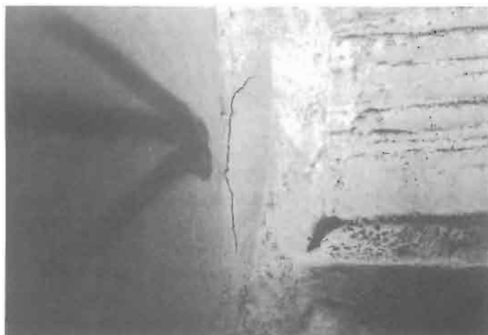
Fig. 5. Typical cracks found at external support welds.
