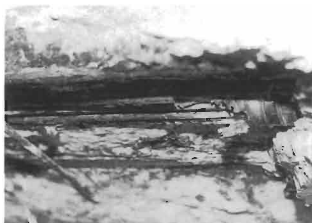
Fig. 3. Corrosion damage of cables.
