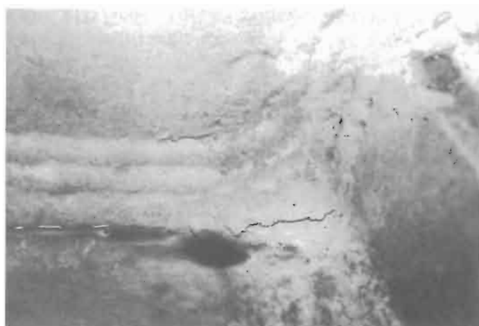
Fig. 6. Typical cracks found at external support welds.
