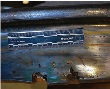
Fig. 68 Top view of damage to area 3 from Fig. 63
