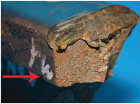
Fig. 96 Fracture surface and wheel impact damage. Red arrow indicates weld material and grinding marks
