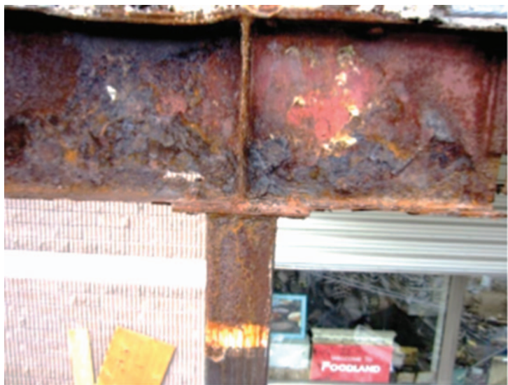
Figure 7-4. Severely corroded connection exposed after the roof collapse. Source: Figure 1.3.5 in Elliot Lake Inquiry (2014) © Queen’s Printer for Ontario, 2014.
