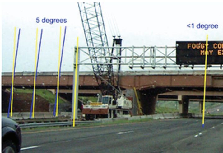
Figure 4-4. Portion of the photograph taken by a driver on May 13, 2004, while the accident girder was in place over I-70.
