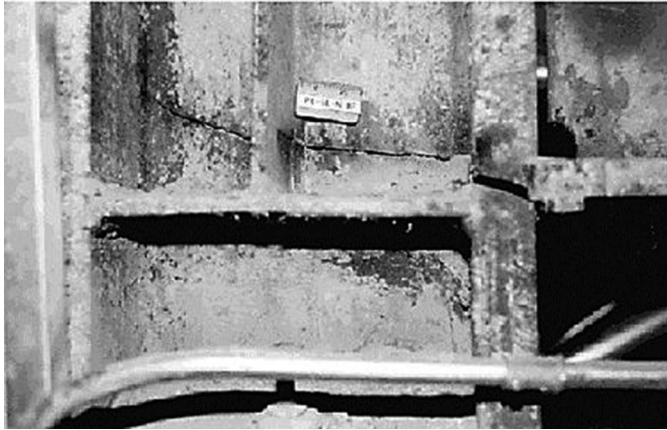
Figure 3-5. Brittle fracture observed after the Northridge Earthquake in a W14 steel column.
