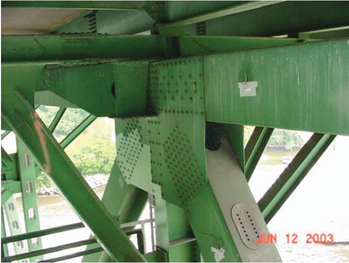
Figure 6-3. Node U10 West before collapse.
