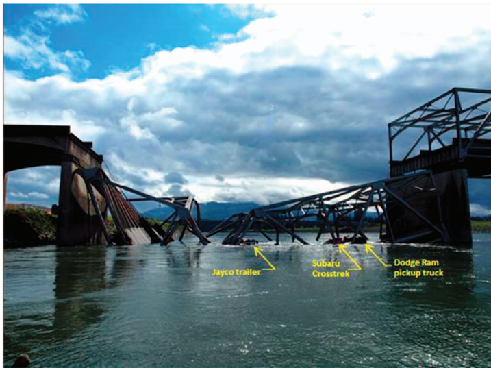
Figure 8-2. Through-truss Span 8 collapsed into the Skagit River.
