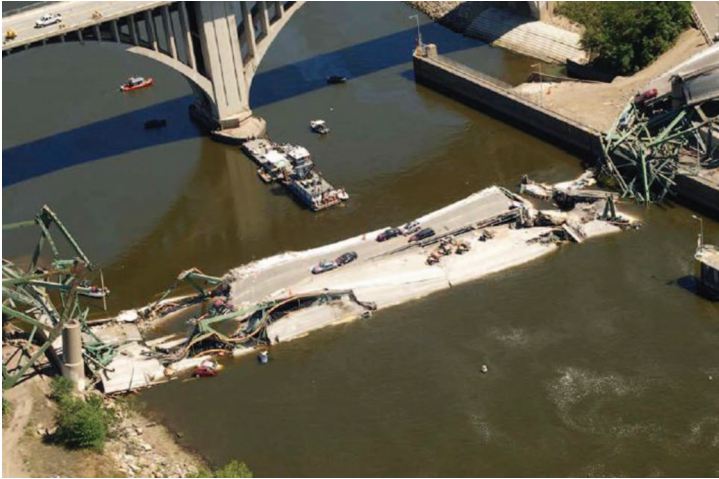
Figure 6-1. Collapsed bridge center section.
