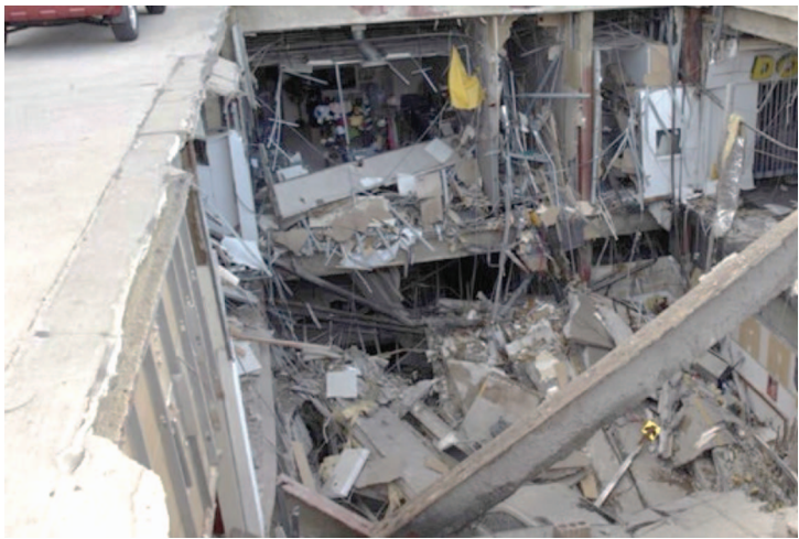
Figure 7-1. Collapse of the rooftop. Source: Figure 2.3.1 in Elliot Lake Inquiry (2014) © Queen’s Printer for Ontario, 2014.
