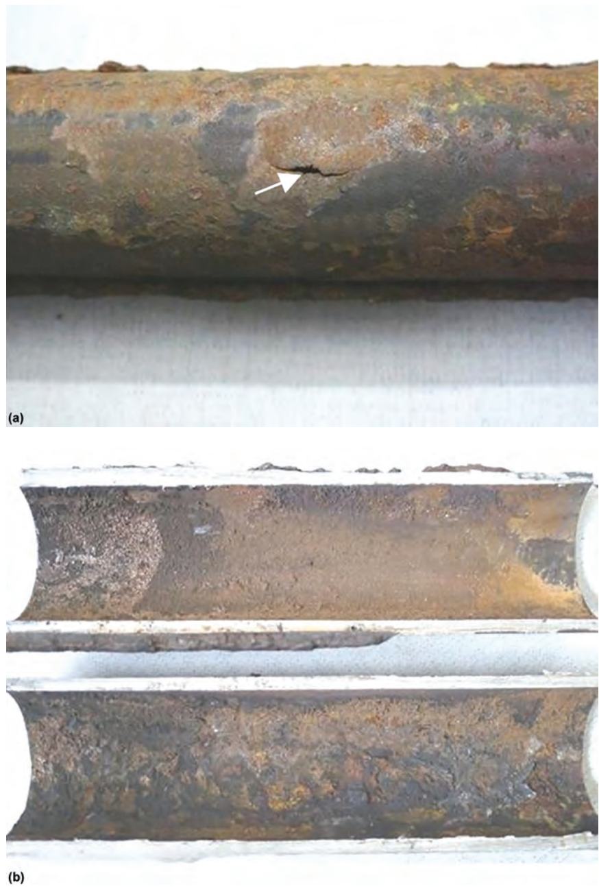
Fig. 6.62 (a) Outer surface of a failed tube sample showing a linear crack. (b) Inner portion of the tube with grayish black scale
