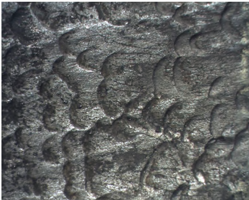
Fig. 6.85 Cavitation damage in a boiler tube
