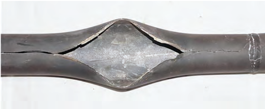
Fig. 6.39 Close-up view at the failure location. The rupture is in the form of a fish-mouth opening. A crack extends in the longitudinal direction from one end of the rupture.
