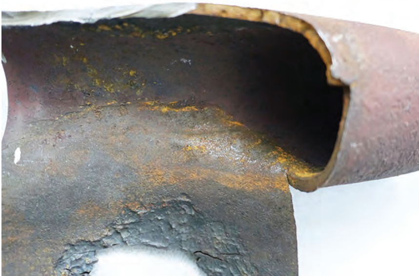
Fig. 6.56 Failed waterwall tube with window opening at tube bend
