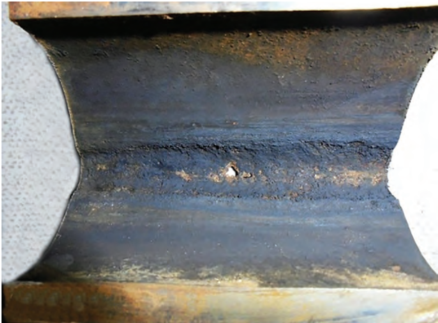
Fig. 6.61 Deep caustic gouging below the insulating deposits on ID side of an economizer tube
