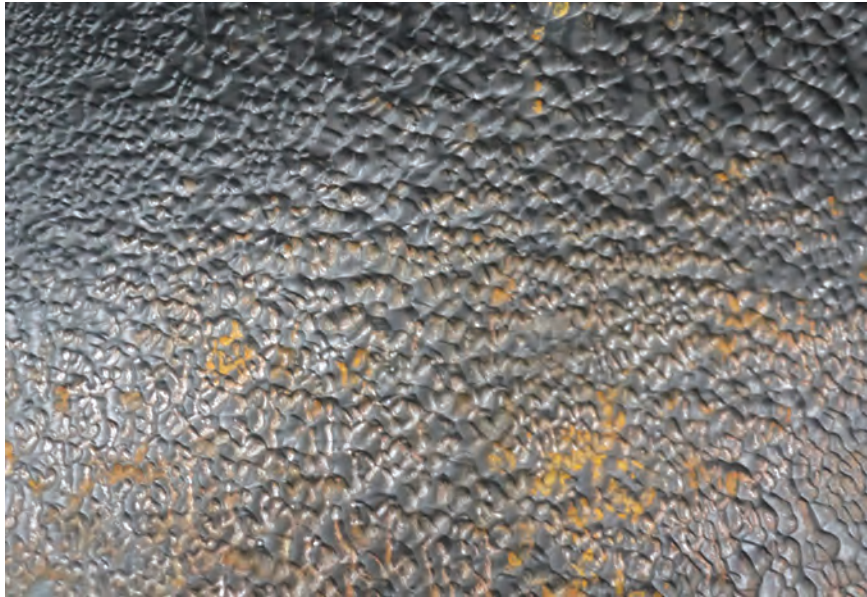
Fig. 6.71 ID surface of a tube showing shiny metal surface with sand-dune-like appearance in the direction of flow due to FAC
