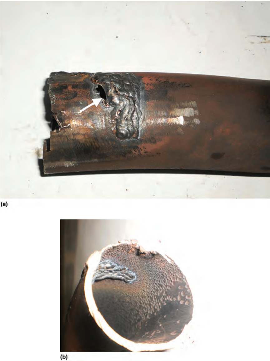
Fig. 6.74 Close-up views of (a) OD side and (b) ID side of the tube bend showing puncture and repair weld area
