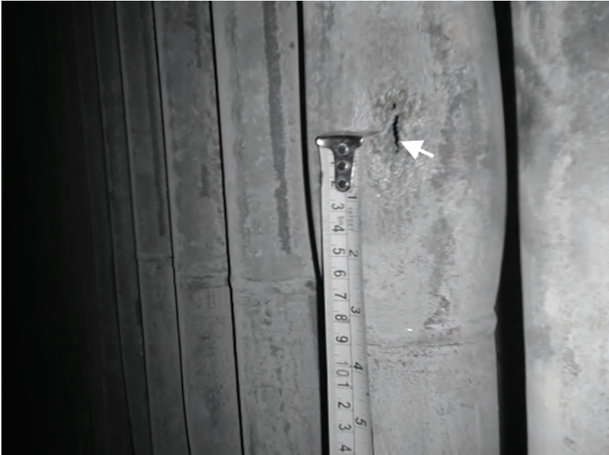
Fig. 6.27 Longitudinal crack in a tube
