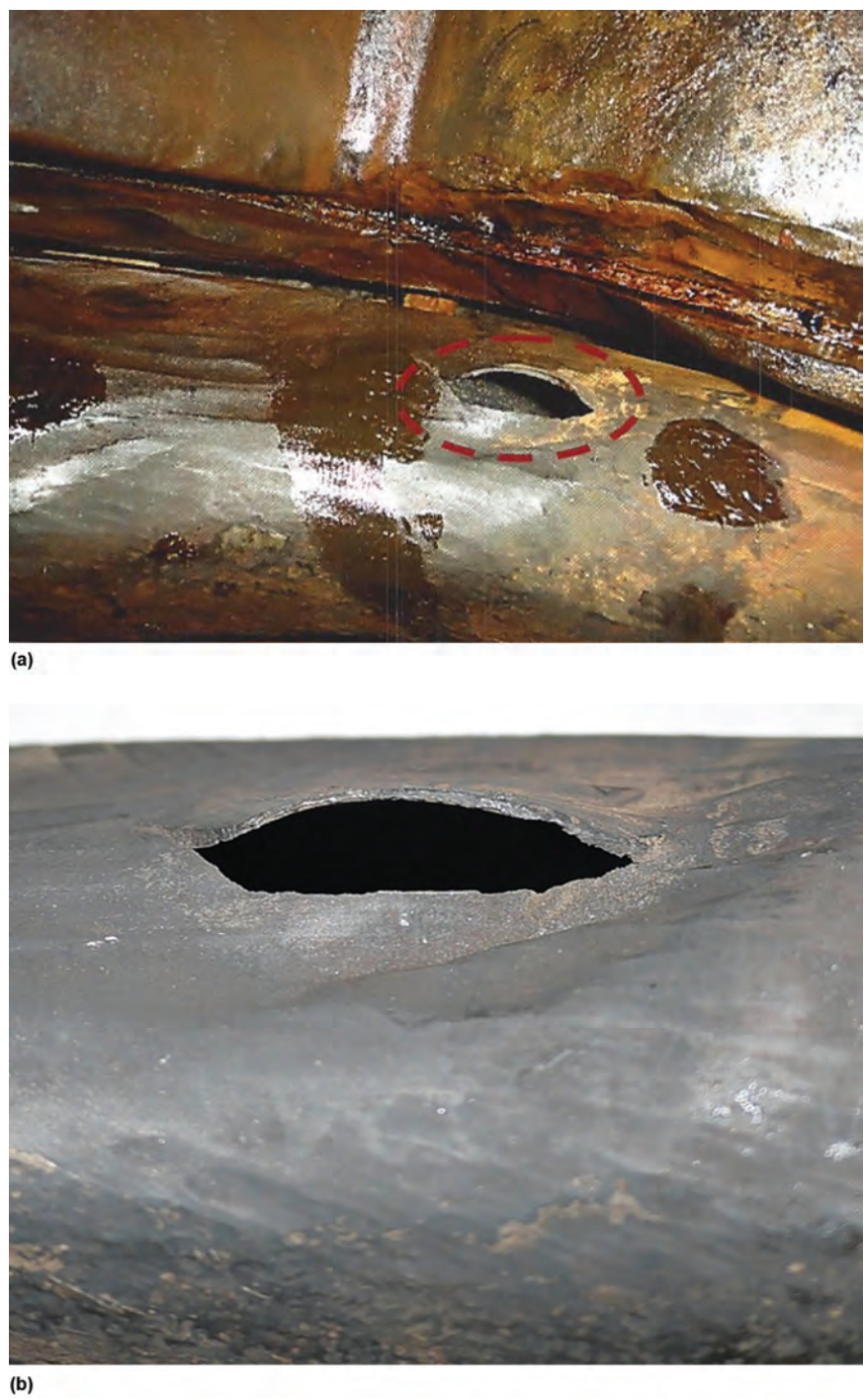
Fig. 6.126 Erosion and longitudinal rupture of boiler tube due to misaligned soot blower
