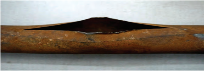
Fig. 6.128 Low-temperature reheater tube showing longitudinal rupture opening
