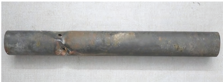
Fig. 6.131 Superheater tube cut by steam leaking from an adjacent tube
