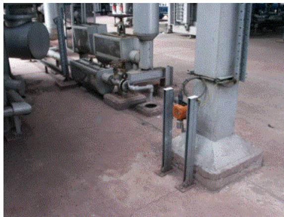
Figure 5.2: Catalytic flammable gas detection in process area
