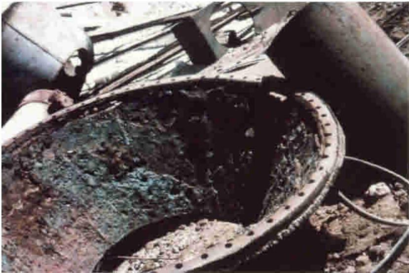
FIGURE 14.9 Corrosion of a CS water box coupled to copper alloy heat exchanger tubes and a tube plate.
