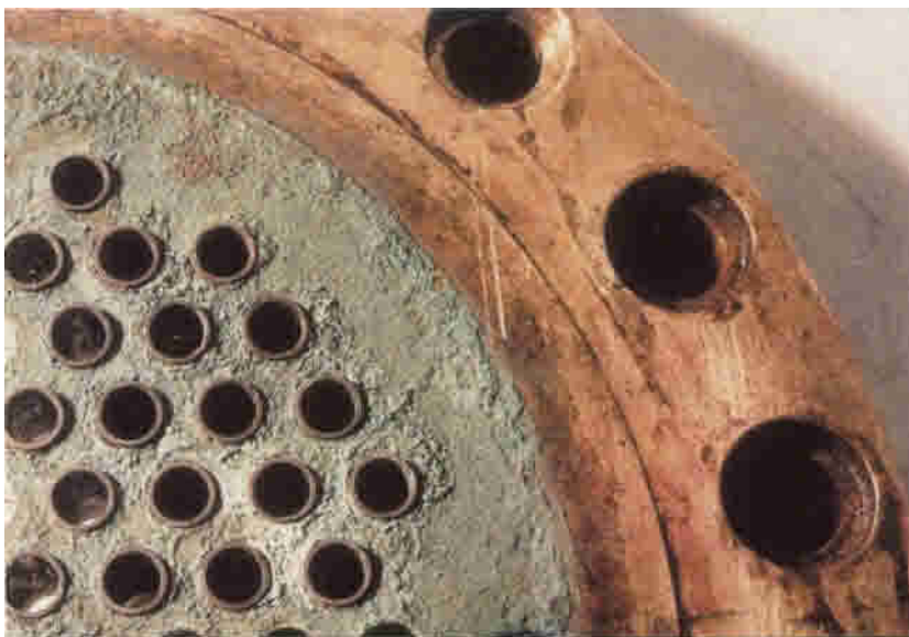
FIGURE 14.5 Galvanic corrosion of a NAB tube plate with titanium tubes.
