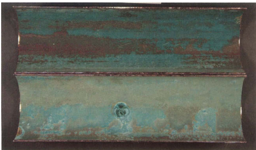
FIGURE 5.3 Type I pitting in a water with high phosphate. (Photograph courtesy of P. Munn.)
