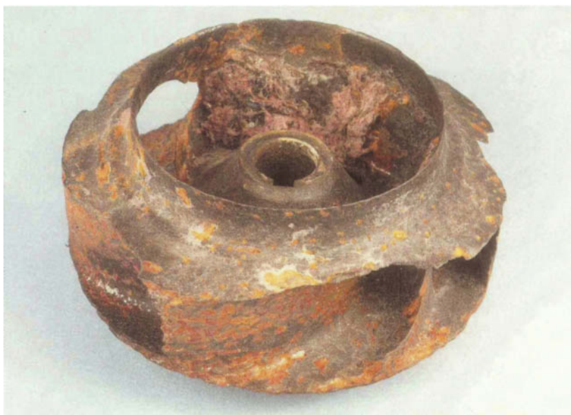
FIGURE 7.29 Severe erosion of a gunmetal impeller due to a high level of suspended solids.
