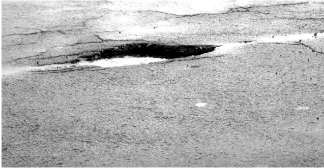
FIGURE 5.1 Rolling contact fatigue of a macadam roadway.
