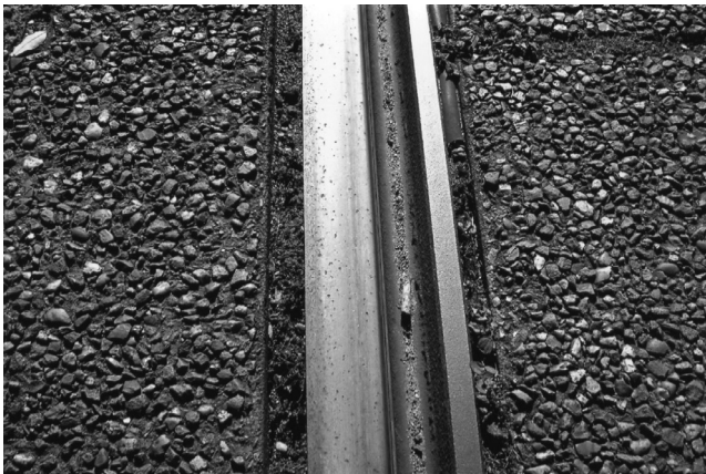
FIGURE 5.3 Pitting on a frequently used tram track.
