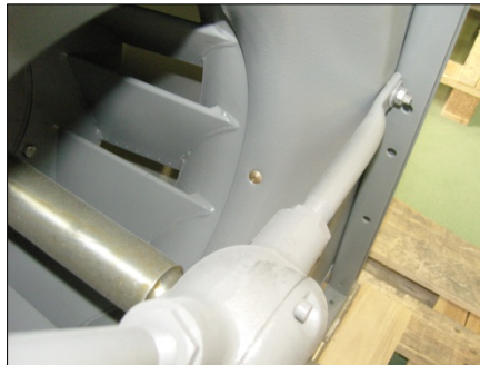
Picture 7 – Pressure measurement orifice in FAN air inlet (external view)
