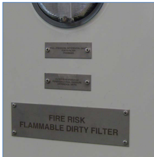
Figure 3 – Names plates under the differential pressure gauge
