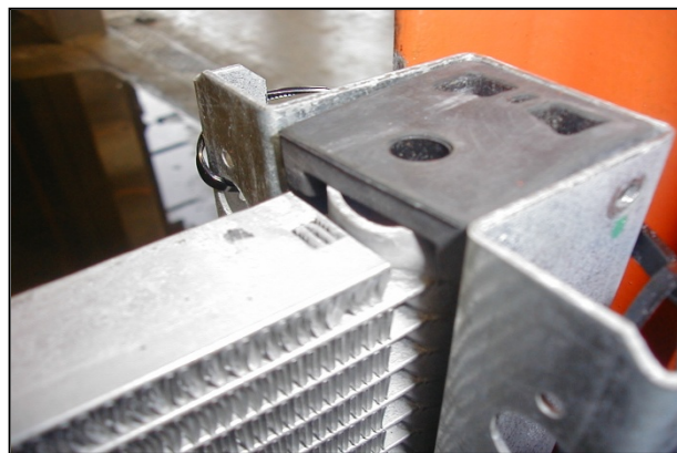
Condenser isolating supports
