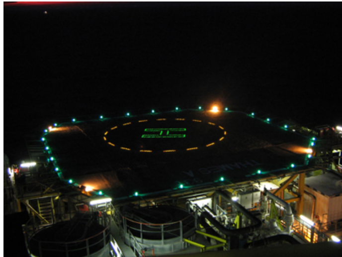
Typical ASPSL lighting system (Helideck Lighting System fitted to North Sea Platform)
