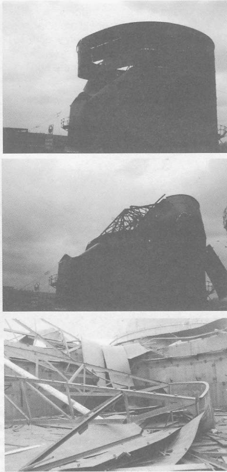
Figure 12.10 Example of severe wind damage to a tank (continued)
