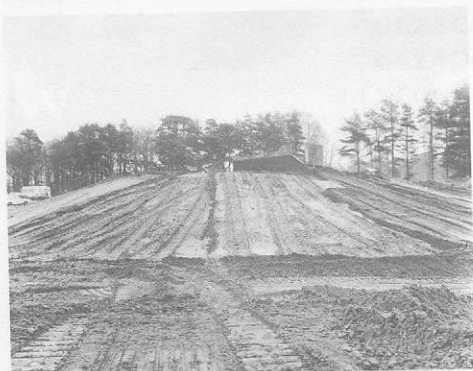
Figure 3.80 The whole structure is partially or completely buried Courtesy of Whessoe
