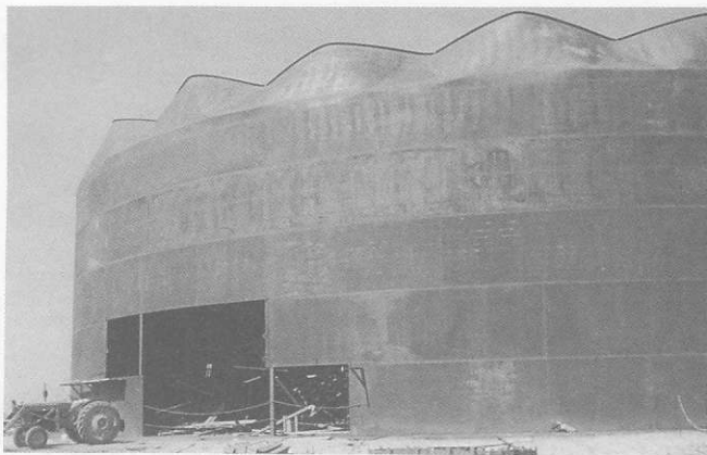
Figure 5.12 A view from outside the tank shell when the roof had failed Courtesy of Whessoe
