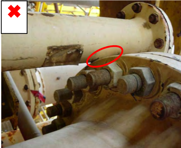
Clash between pipes resulting in fretting damage
