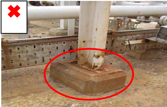
Concrete pipe support plinth detached from ground
