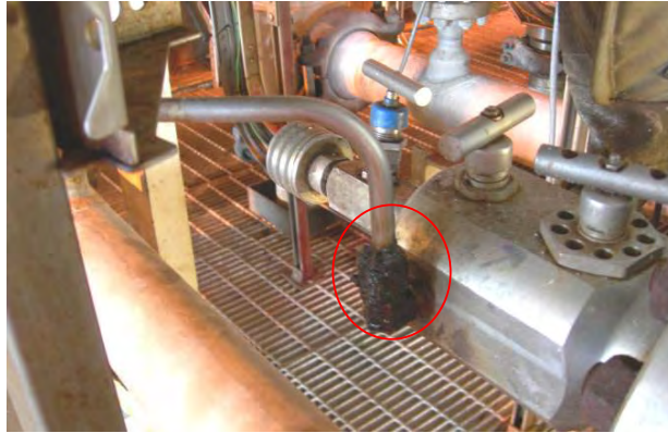
Figure T6-5 Example of weeping at the tubing connection
