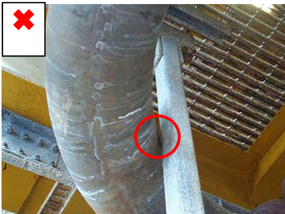
Pipeline contact to cable rack resulting in fretting damage
