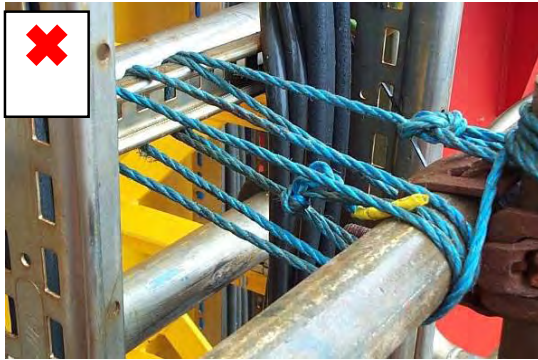
Rope used to support cable tray
