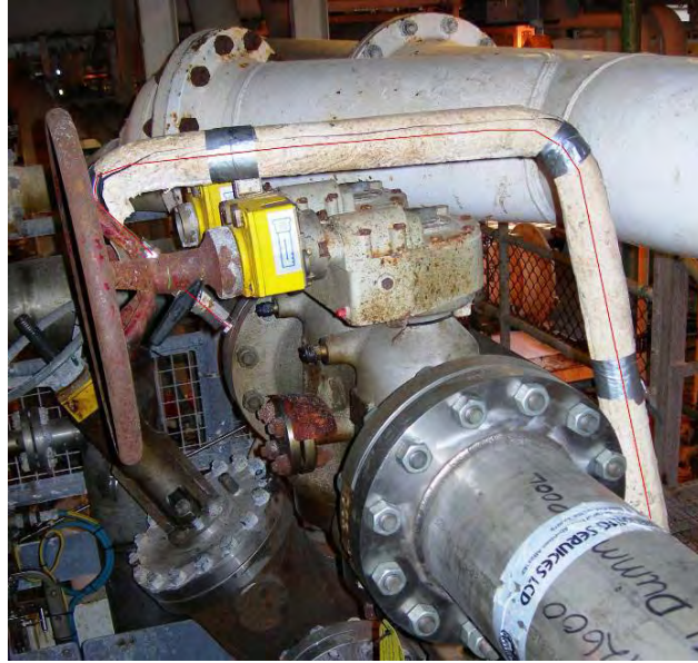
Figure T6-6 Example of disconnected tubing which has not been supported
