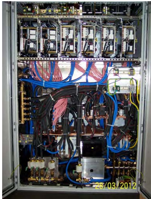
Figure 6.27: Converter and resonant circuit of a 300 kW SDF ® generator (Source: eldec)
