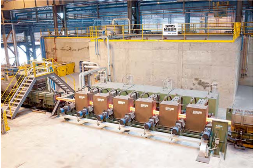
Figure 2.24: Induction heating plant with 6 induction coils at Tung Ho Steel in Taiwan (Source: SMS Elotherm)
