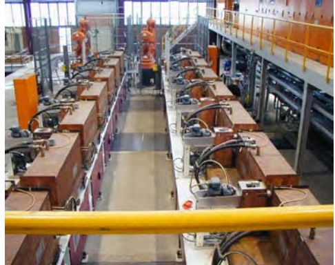
Figure 2.14: Induction heating plant in a forging line for billets (Source: SMS Elotherm)
