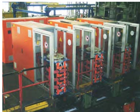
Figure 2.53: Re-heating plant with 3 individual coils and 4 control zones each (Source: IAS GmbH)
