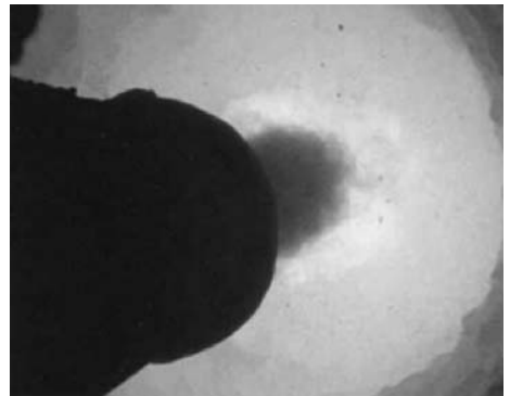
Flame following correction of secondary air flow patterns
