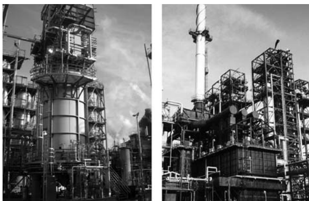
Figure I.24 Two types of refinery heater showing a cylindrical heater (left) and a cabin heater (photos provided courtesy of Born Heaters, Canada, an Onquest company)
