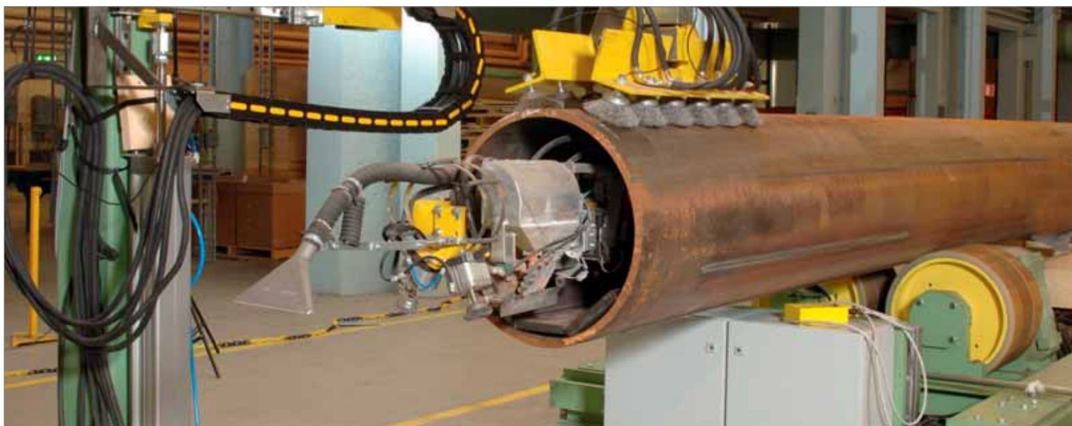
Figure 4. Current return system with steel brushes on top of the pipe.
