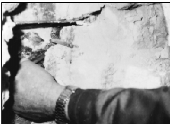
Fig. 2800-7 Secondary Reformer Vessel— Large void exposing back-up layer of two-component lining. Replace hot face and back-up layers and re-weld any anchors that come loose during refractory removal.
