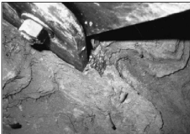
Fig. 2800-6 FCCU Regenerator, Below Grid— Laminated refractory and non-distributed metal fibers means poorly mixed material at installation time. Photo taken after 3 years of service. Replace both refractory and anchorage.
