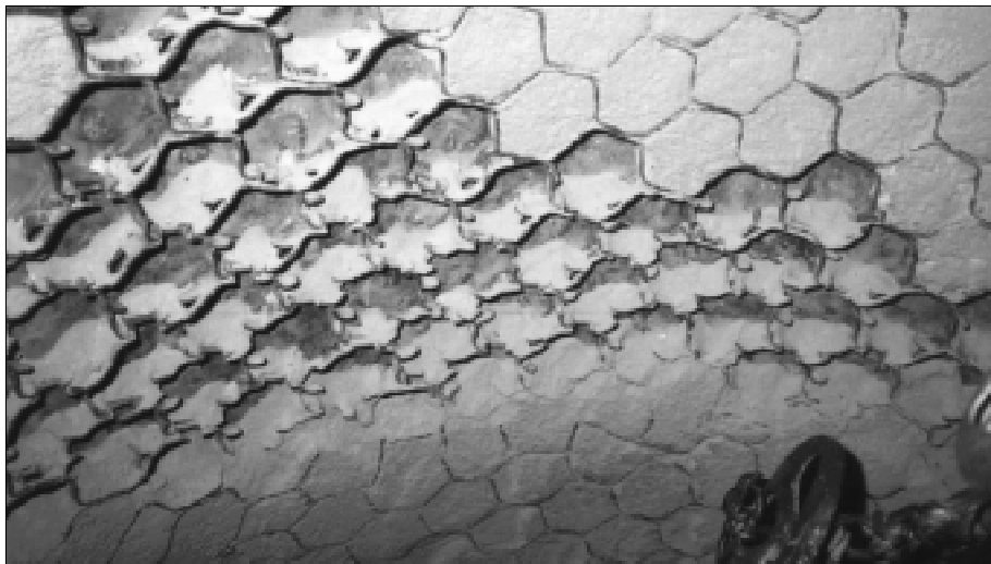
Fig. 2800-2 FCCU Cyclone— Refractory and hexmesh have washed out. Metal has eroded down to the lances and clinches. Replace both hexmesh and refractory.
