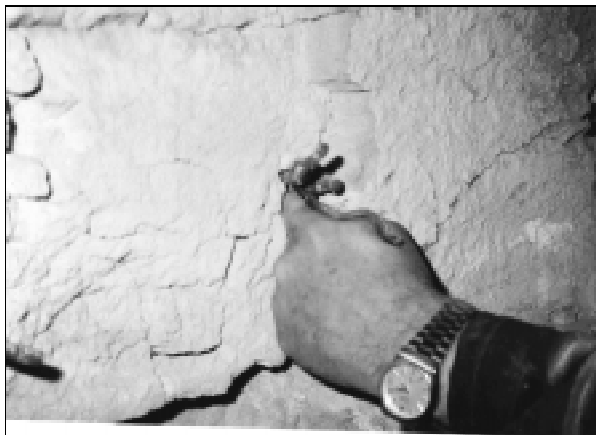
Fig. 2800-8 Secondary Reformer Vessel— Hot spot at anchor void just below vapor stop ring. Replace hot face and back-up layers and re-weld any anchors that come loose during refractory removal.
