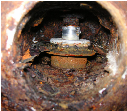
Figure 17.3.4-1: Symptom 12 - Strong corrosion in a safety valve
