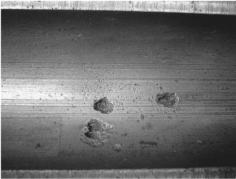
FIGURE 7.5 Pitting corrosion on the inside surface of a steam condensate pipe.
