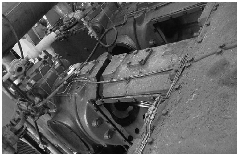
FIGURE 14.7 Reciprocating compressor casing damaged by a broken bolt.
