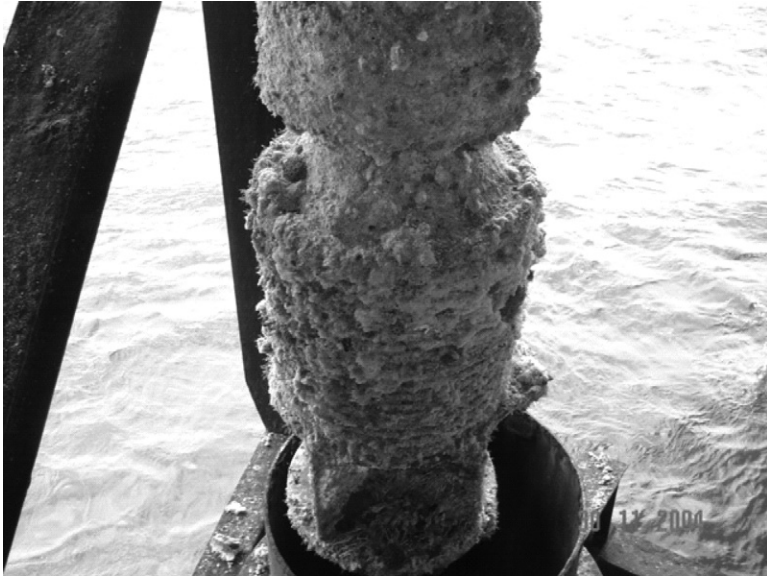
FIGURE 8.8 Seawater pump suction strainer with heavy biological incrustation.
