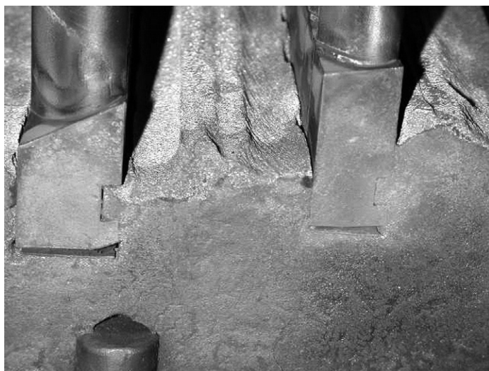
FIGURE 6.21 Erosion on a steam turbine casing.
