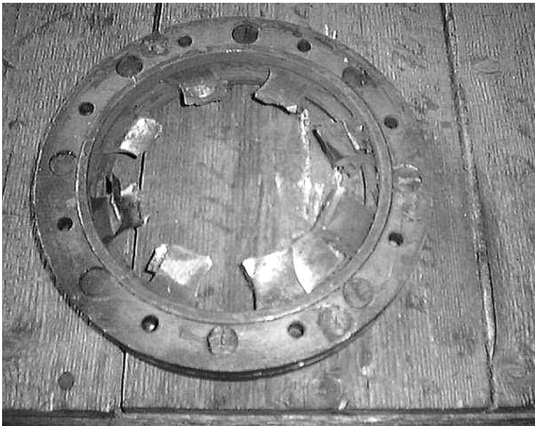
FIGURE 18.2 Cooling tower fan coupling elastic element displaying fatigue failure due to misalignment.
