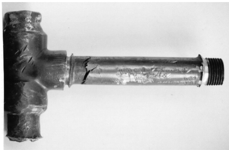
FIGURE 7.12 Drain piping with stress corrosion cracks.
