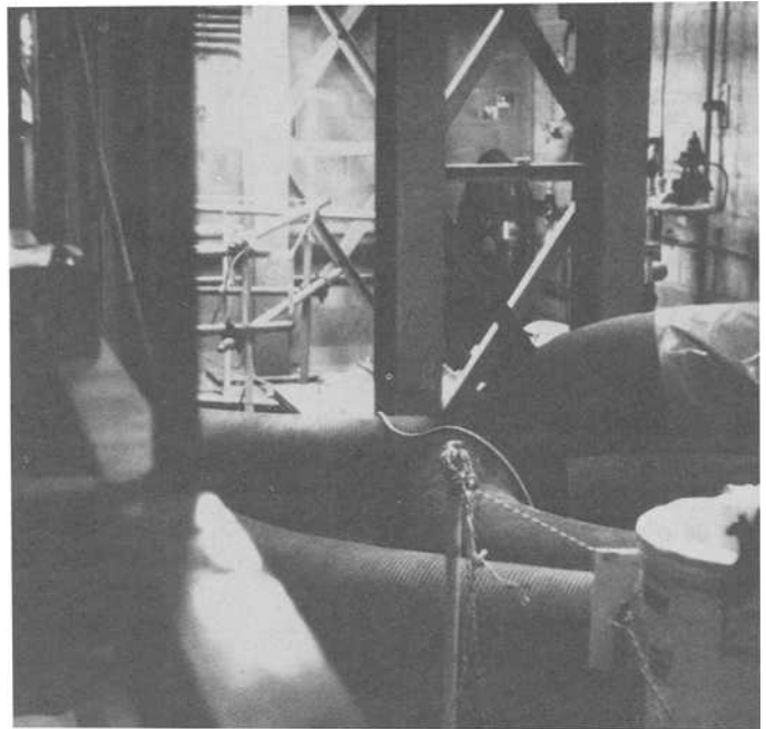
FIG. 5—Torus coating ventilation ducting (courtesy of Iowa Electric Light and Power Co.).
