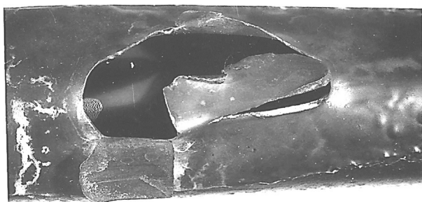
Fig. 11.2.3 Thinning of the failed region seen on the tube.
