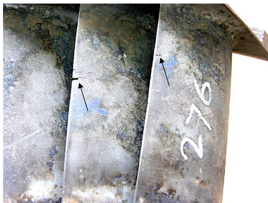
Fig. 12.5.2 Close-up view of one segment of the vanes showing cracks near the trailing edge on the convex side of the aerofoil.
