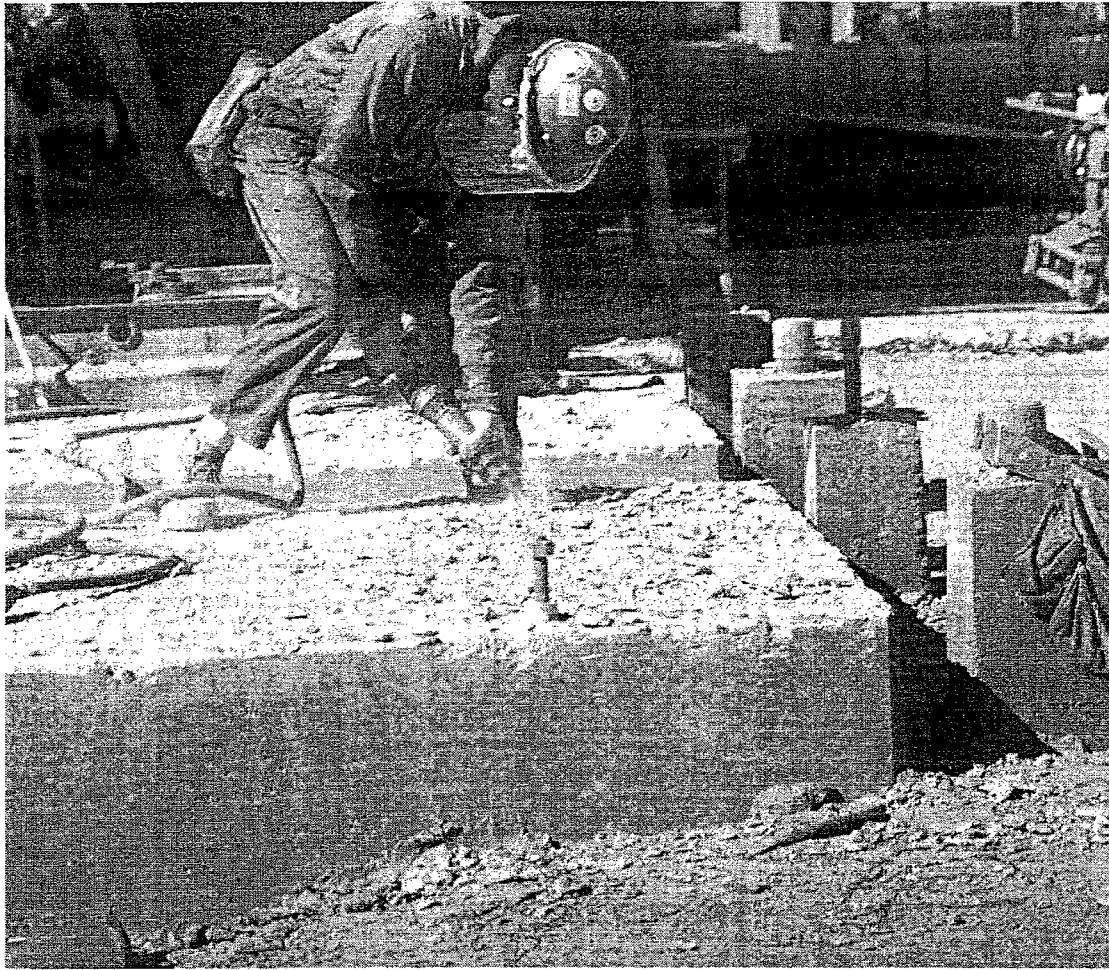
Figure 3-48. Chipping of concrete foundation.
