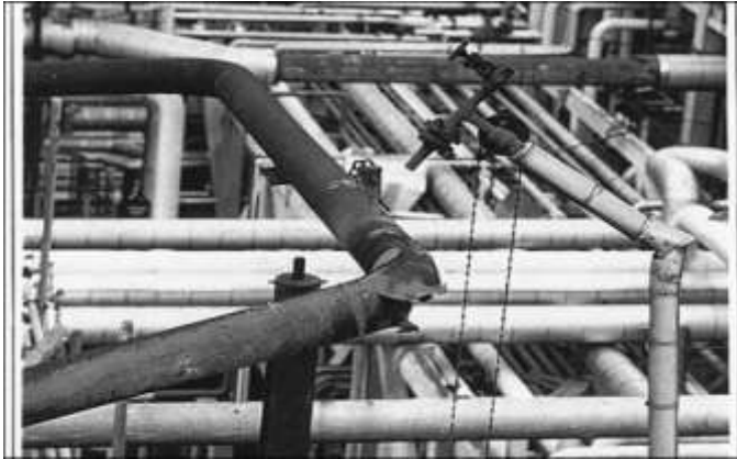
Figure B5b: Failure Downstream from Intermittent Injection Point
