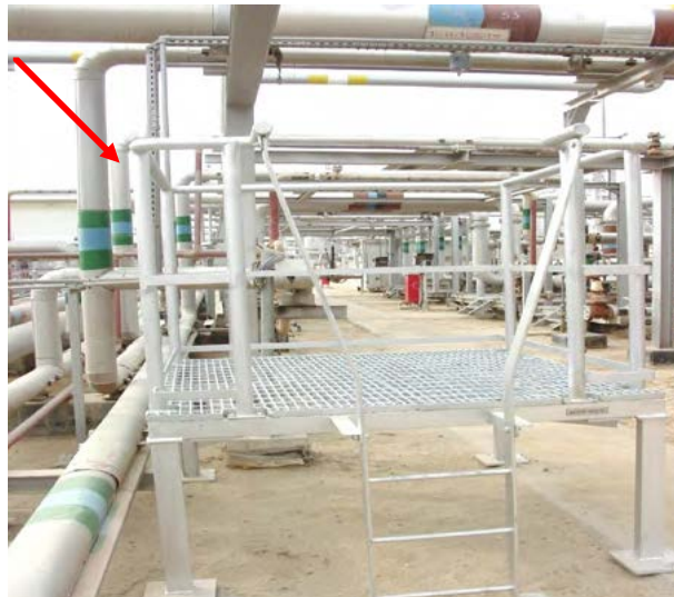
Figure 9D: Permanent Access Platform
