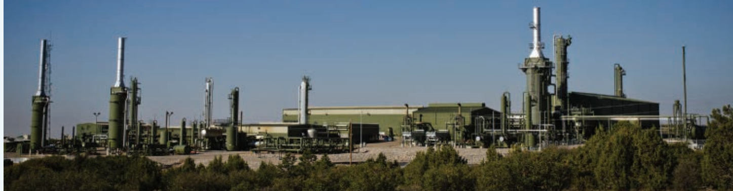
▼ Red Cedar's Coyote Gulch gas plant on Southern Ute reservation in San Juan basin.
