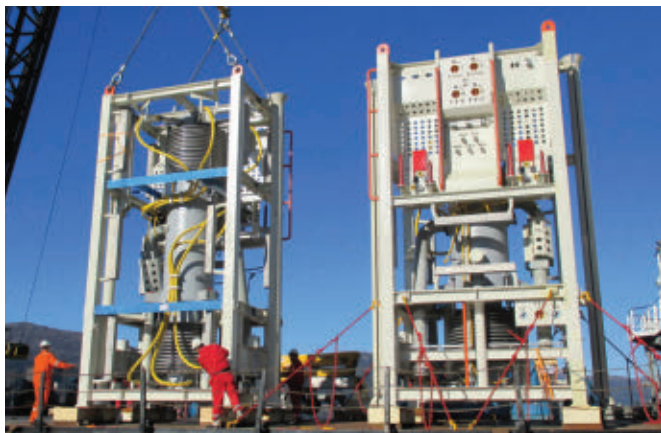
Two multiphase compressor units at the OneSubsea facility in Horsøy, Norway. (Photo courtesy OneSubsea)
