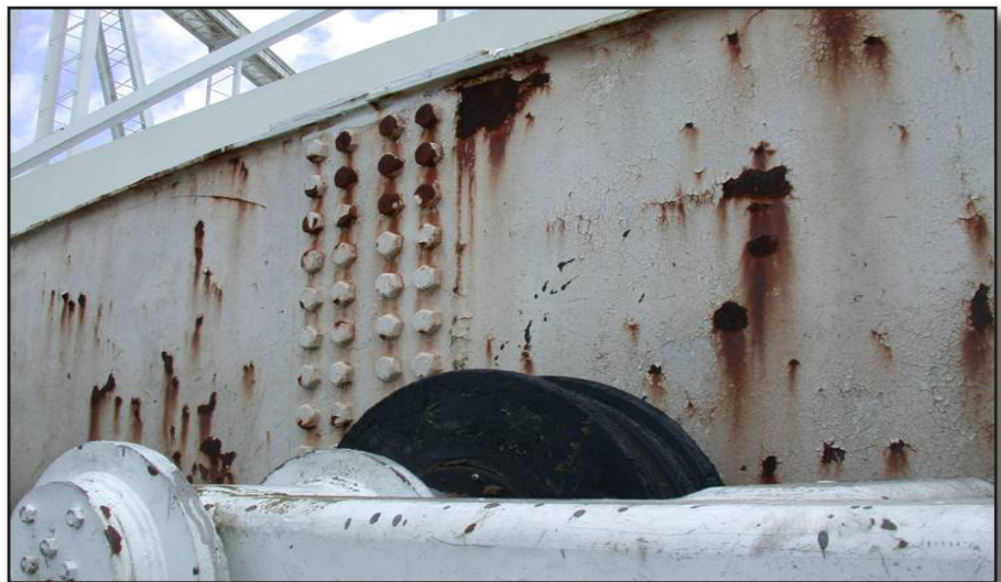
Corrosion in Process
