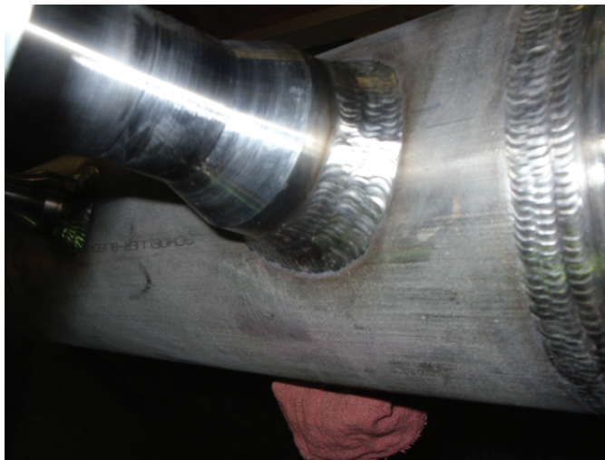
Figure 2.12.12 Typical stainless-steel pipe weld, and weld-o-let on the header.
