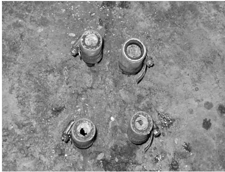
Fig. 3.8 Calcium-clogged water paths due to high-conductivity water. Source: Ref 7
