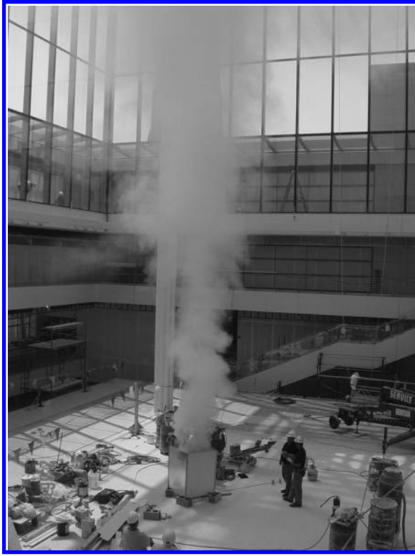
Figure 10.4 Smoke test in atrium. (Image courtesy of Jensen Hughes.)
