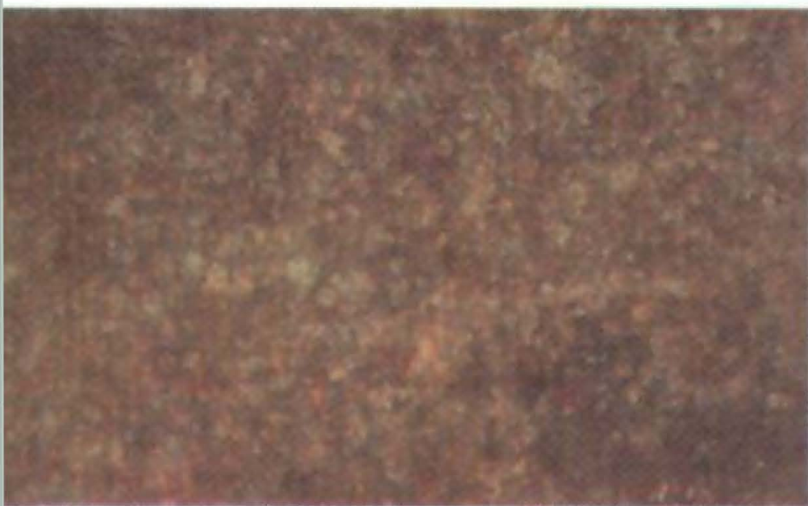
Rust Grade C
