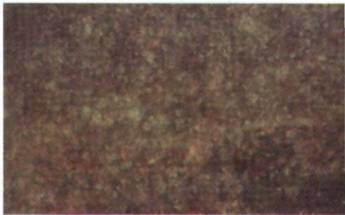
Rust Grade C
