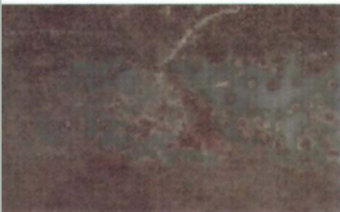
Rust Grade B
