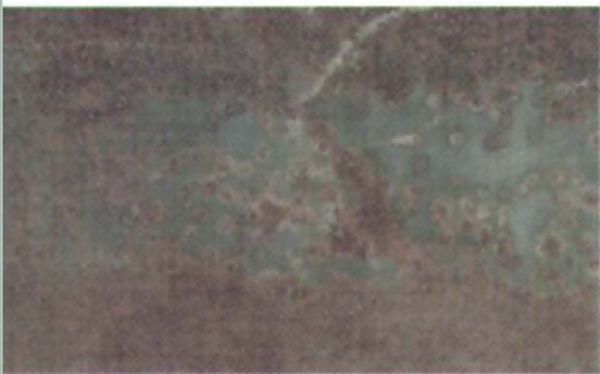
Rust Grade B
