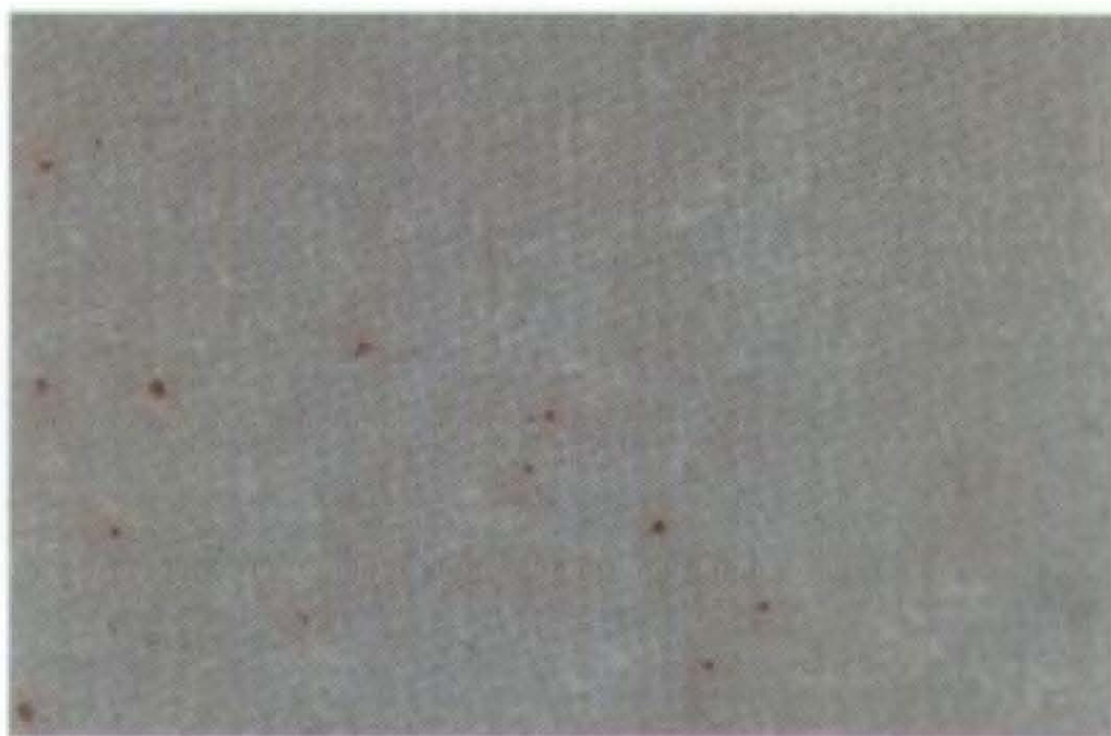
Rust Grade 8-P, 0.1% Rusted
