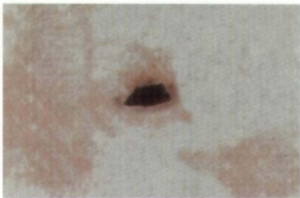
Rust Grade 6-S, 1% Rusted
