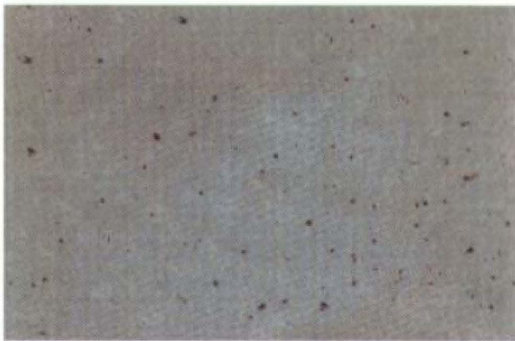
Rust Grade 7-P, 0.3% Rusted
