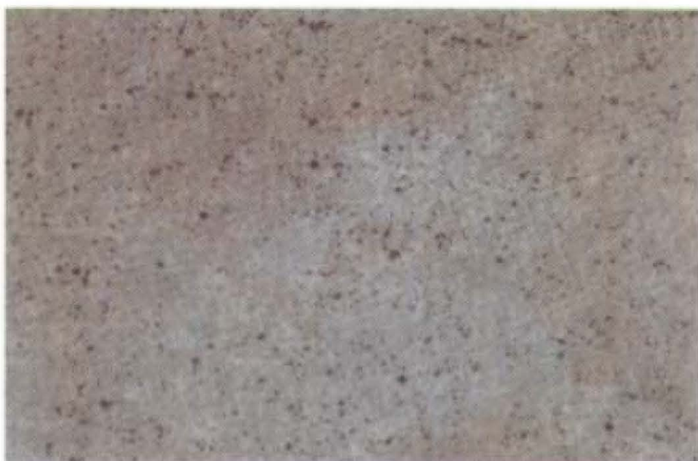
Rust Grade 5-P, 3% Rusted
