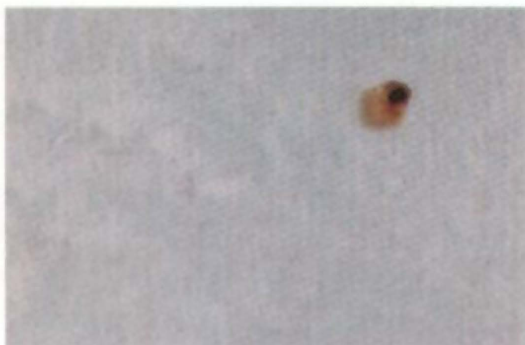
Rust Grade 8-S, 0.1% Rusted
