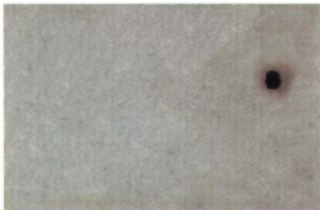
Rust Grade 7-S, 0.3% Rusted
