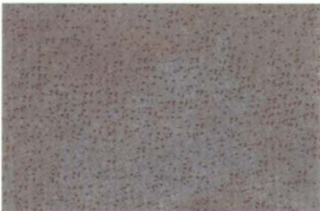
Rust Grade 4-P, 10% Rusted
