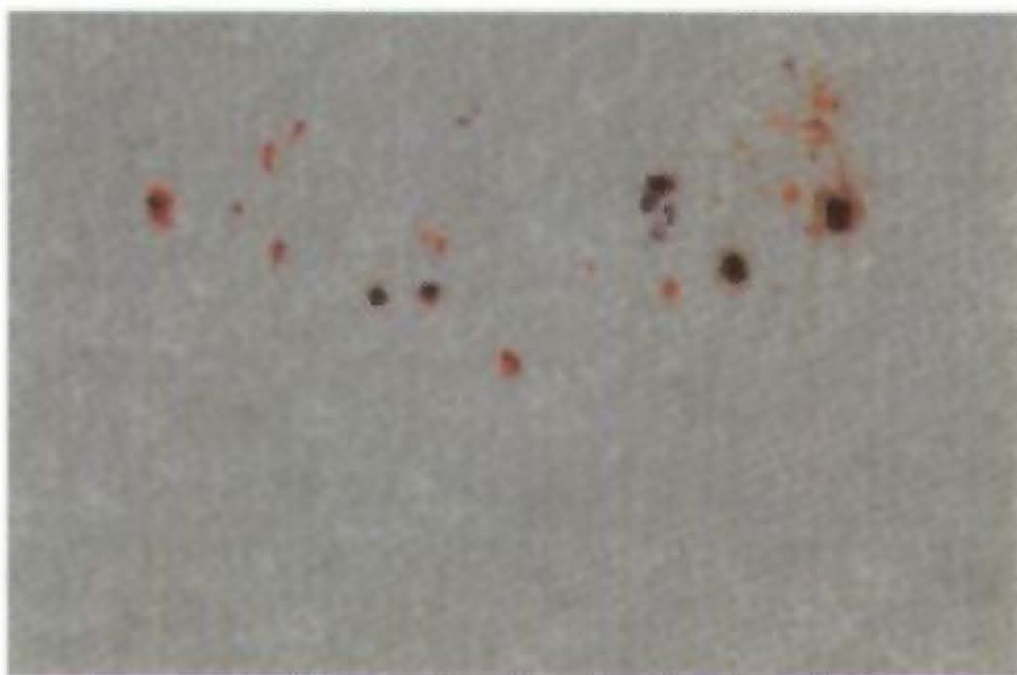
Rust Grade 7-G, 0.3% Rusted
