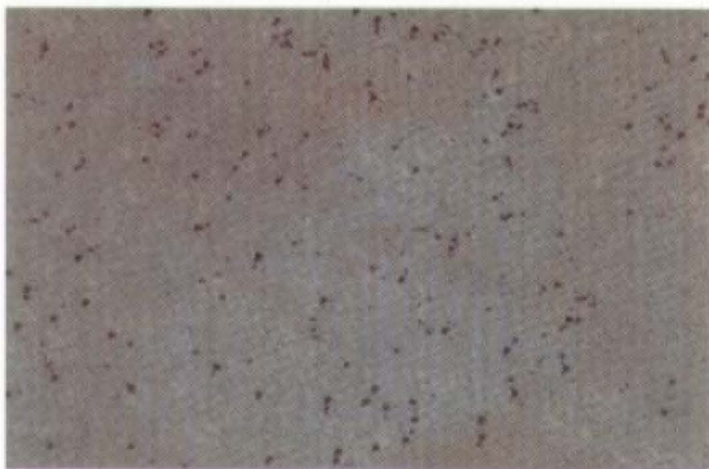
Rust Grade 6-P, 1% Rusted
