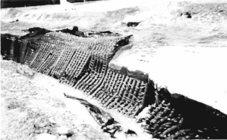
FIG. 1— Deformed and collapsed units.
