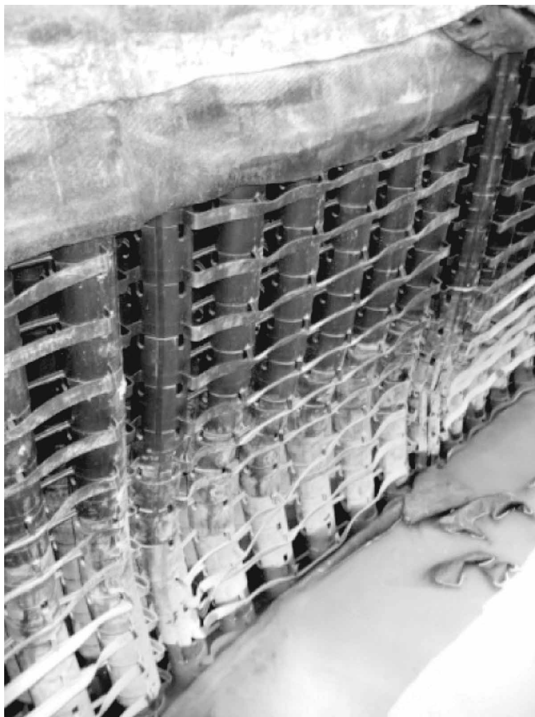
FIG. 2— Lateral deformation at perimeter units.
