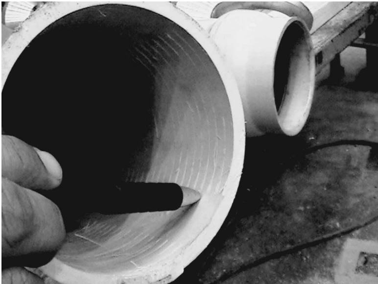
FIG. 12—Indentations left on the internal diameter of the pipe.
