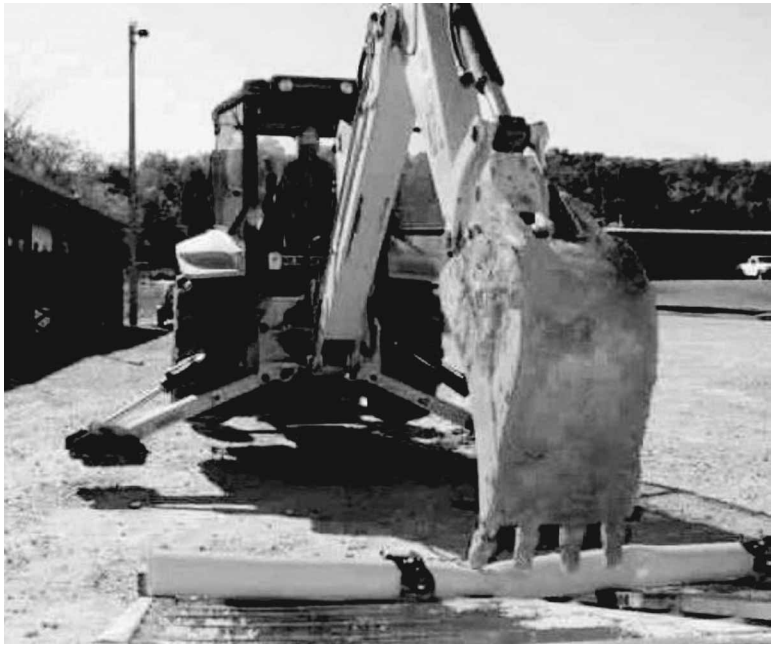
FIG. 12—No puncture of backhoe tooth. Note entire backhoe, wheels and all, off the ground.
