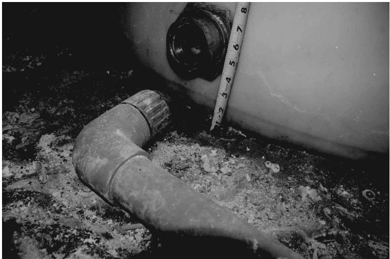
FIG. 20—Failed connection of threaded PVC fitting to acid storage tank.
