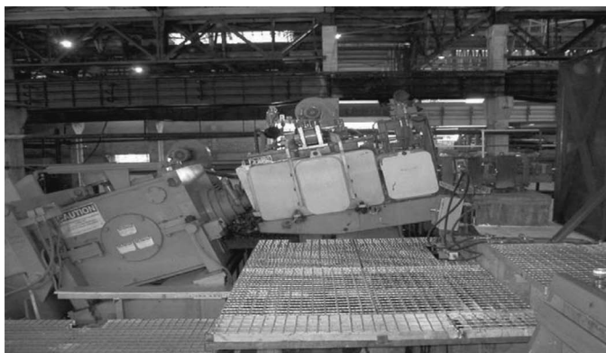
Fig. 14.10 Inclined Pinch Roll & Laying Head.
