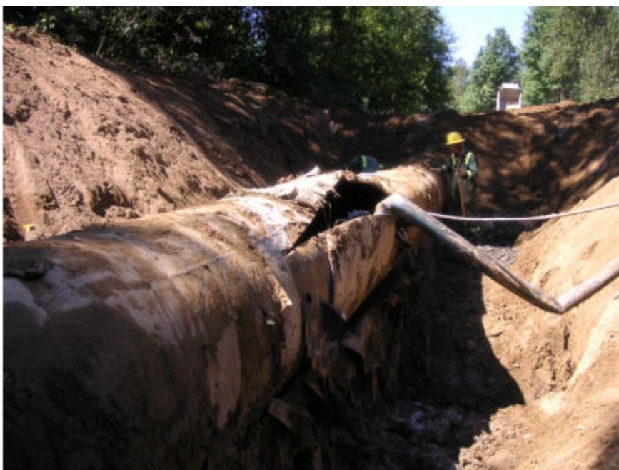
Figure 9.5: Excavated Hydrostatic Test Failure
