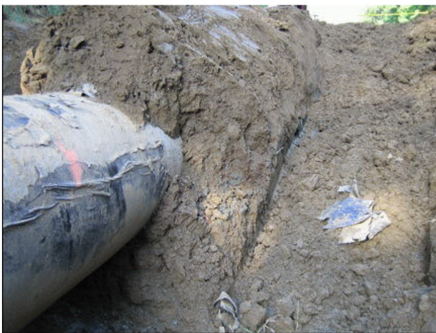
Figure 4.3: Polyethylene tape coating showing evidence of disbondment
