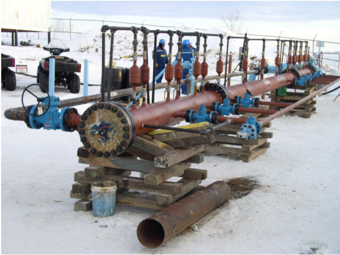
Figure 6.2: Pig launching barrel equipped with manifold to run 'liquid slug' in a natural gas pipeline
