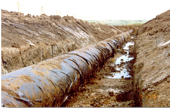
Figure 5.2: Disbonded polyethylene tape
