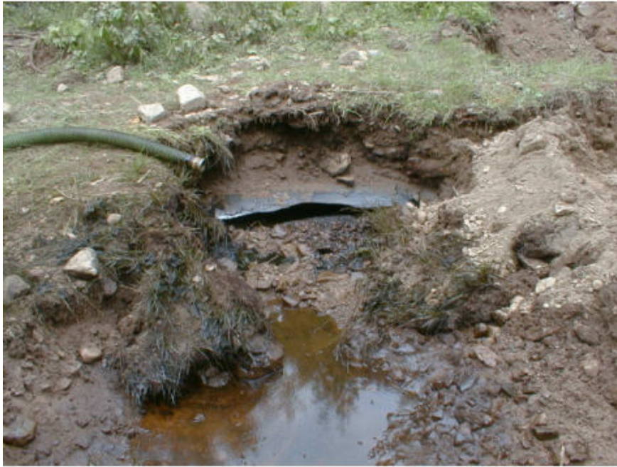
Figure 9.6: Hydrostatic SCC Failure
