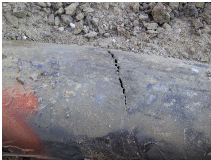
Figure 7.4: Circumferentially-oriented cracks that resulted in a natural gas leak in NPS 8 pipe
