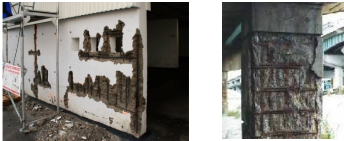
Figure 1: Corrosion of transverse rebars.
