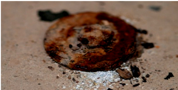
Figure 4: Galvanic corrosion in Scorpion.
