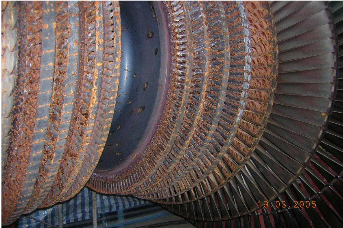
Figure 5: Corroded turbine after salt intrusion and insufficient conservation.
