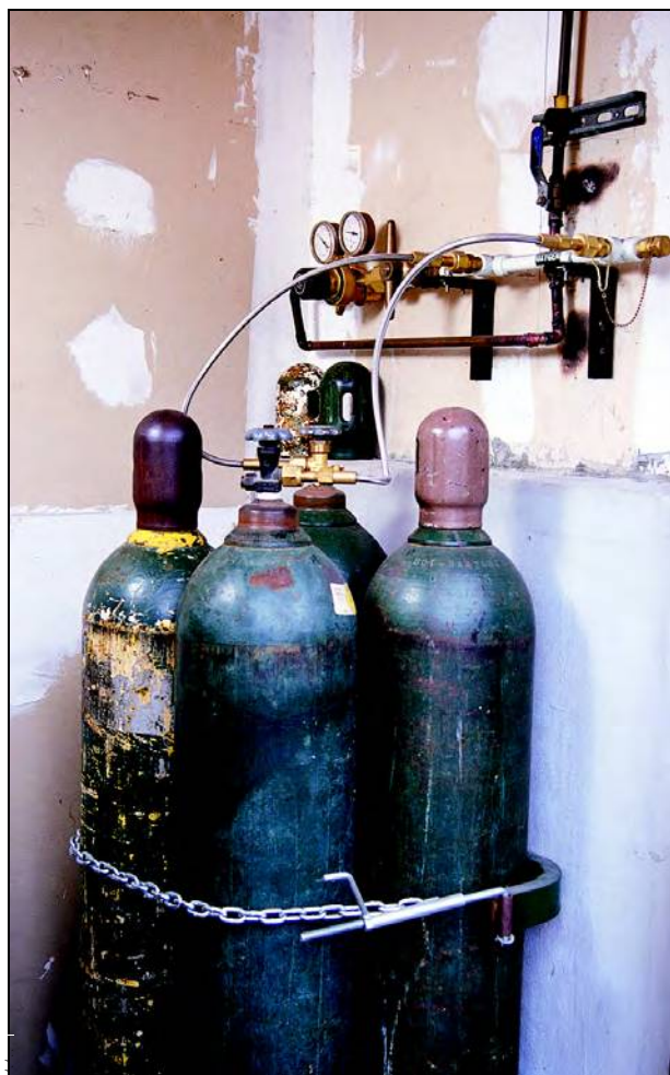
Figure 2.13—Oxygen Manifold System
