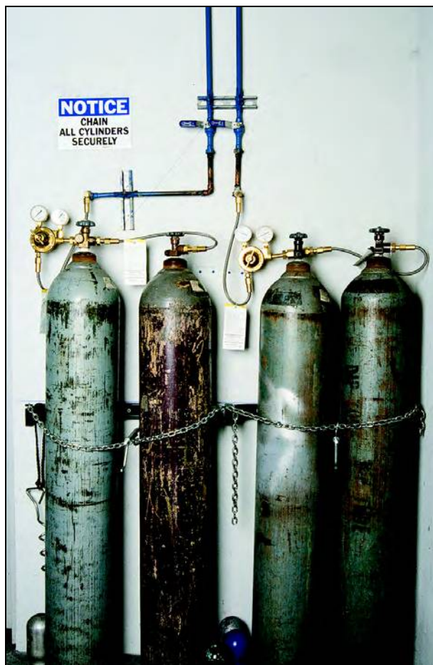
Figure 2.10—Inert Gas Cylinders Attached to Manifold System
