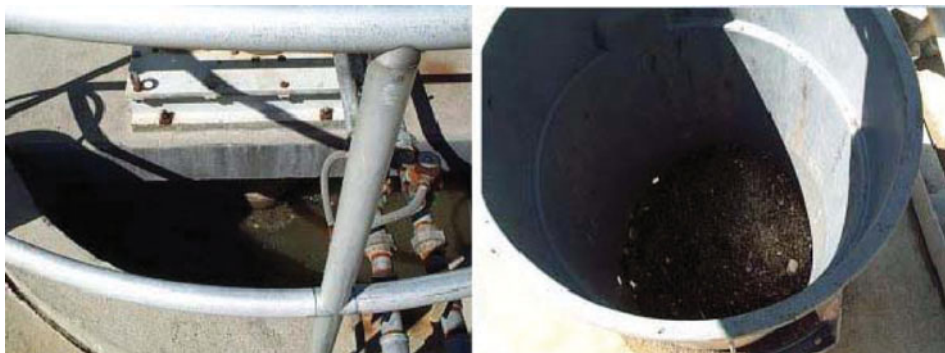
Figure 7.3 Grit chamber (Reproduced with permission from © DDM Imagery).
