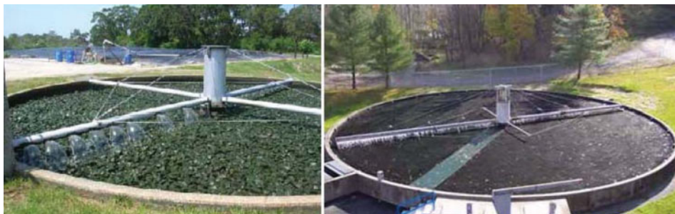
Figure 4.8 Trickling-filter (Reproduced with permission from © DDM Imagery).
