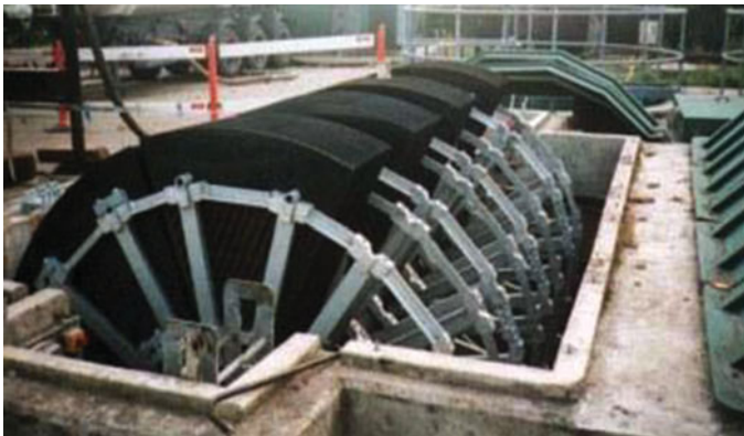
Figure 4.11 Rotating biological contactor (Reproduced with permission from © DDM Imagery).
