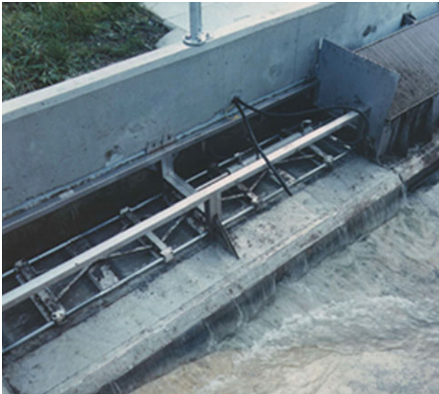
Figure 2.2 A typical bar screen that consists of a series of parallel bars or a perforated screen placed in a channel (Courtesy of City of Phoenix (Arizona) Water Services Department).
