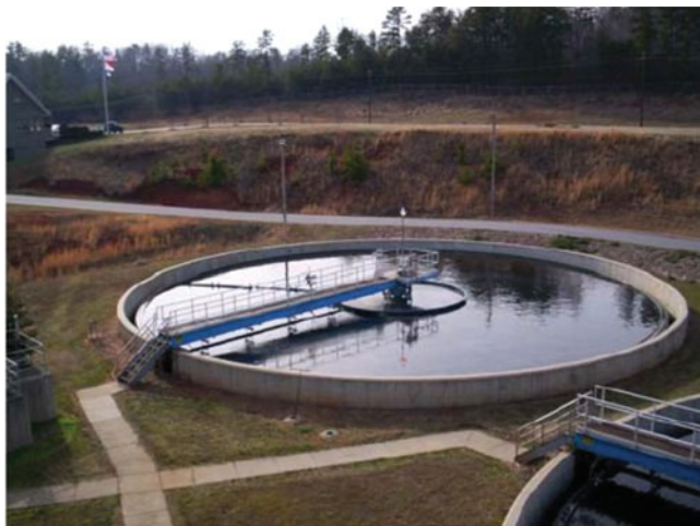
Figure 3.4 Secondary circular clarifier (Reproduced with permission from © Hickory wastewater treatment).
