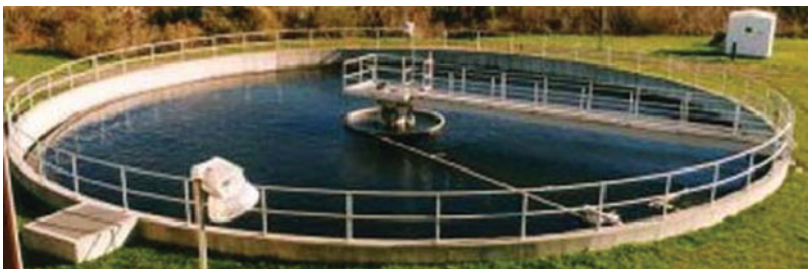
Figure 7.7 Secondary settling tank (Reproduced with permission from © DDM Imagery).
