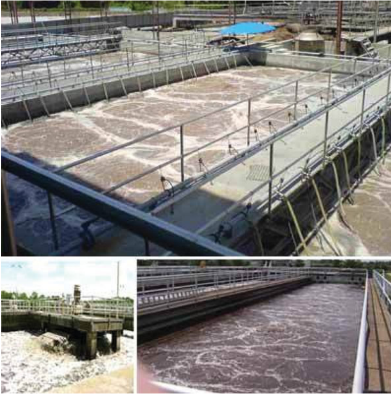
Figure 7.2 Sewage treatment plants (Reproduced with permission from © Shutterstock).
