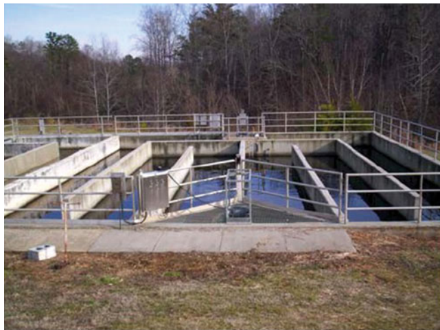
Figure 3.5 Chlorine contact chamber (Reproduced with permission from © Hickory wastewater treatment).
