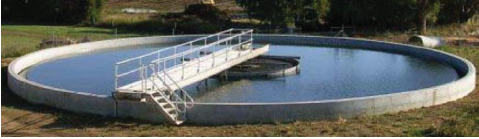
Figure 7.4 Primary settling tank (Reproduced with permission from © DDM Imagery).
