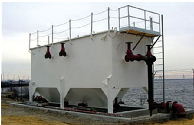
Figure 2.5 A highland rectangular API Oil water separator (Reproduced with permission from © Can-Am Instruments Ltd).
