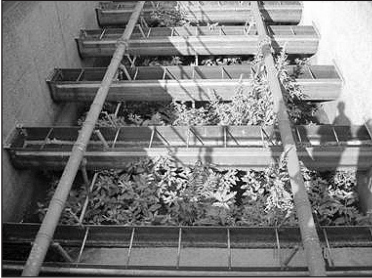
Figure 15-1 An out-of-service filter in an active plant
